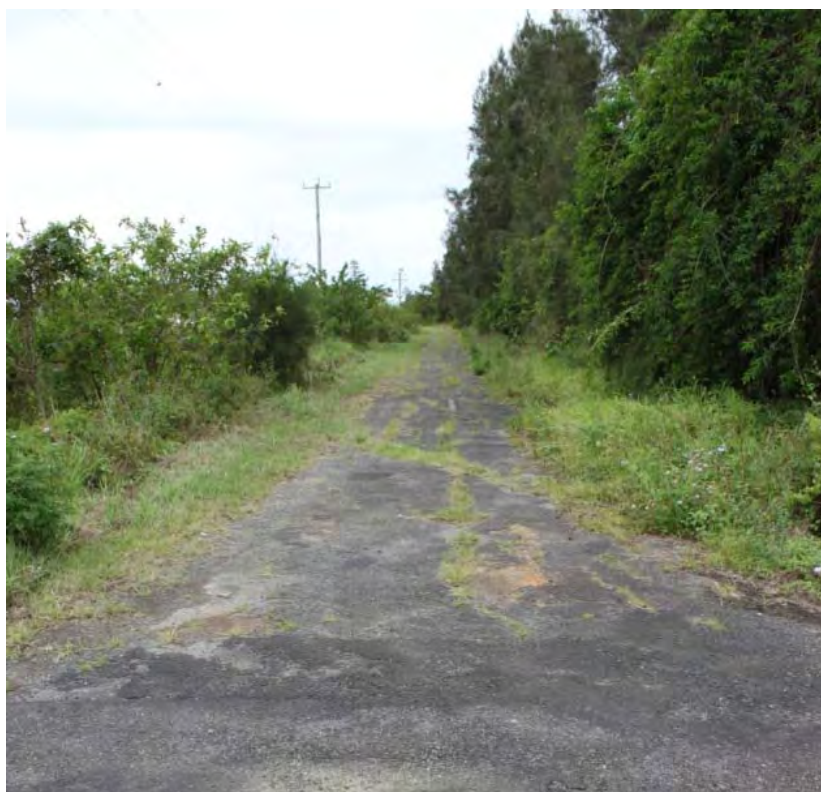
Figure 3-6: Remnants of earlier route of Pacific Highway, northern end of Morpeth Street, Harwood, facing north, photo taken by Rachael Loizou on 28 October 2011.
