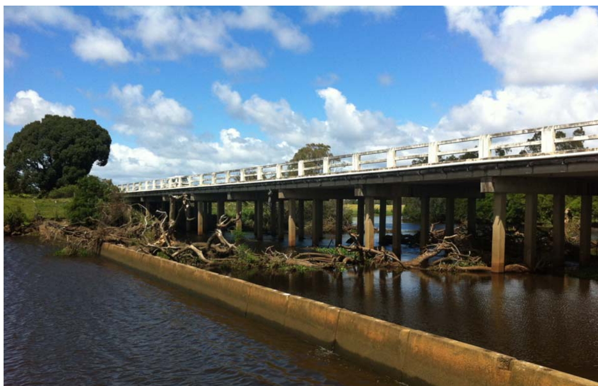
Plate 6-1 Debris blockage at the existing bridge over Tuckombil Canal
