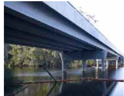
Bridge designs are to be simple with a dominant superstructure. RTA Image
