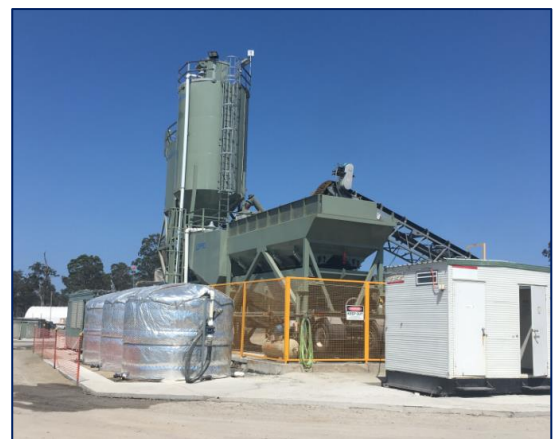
Temporary batch plant at Avenue Road, Pillar Valley for the Woolgoolga to Ballina Pacific
