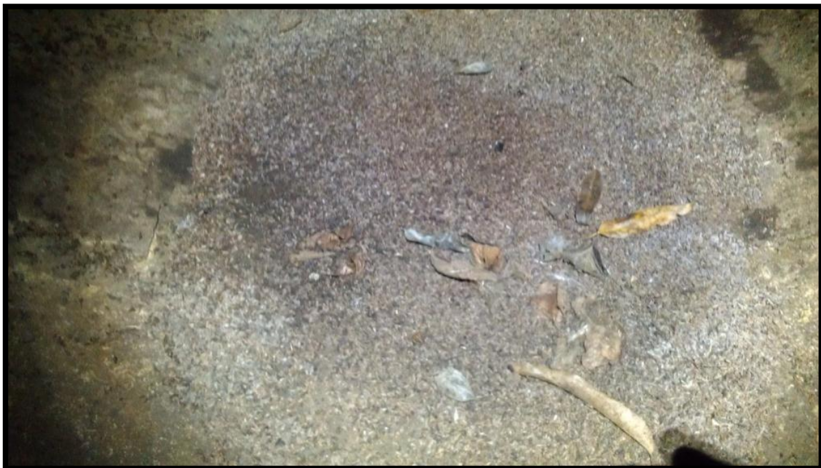
Plate 2-3. Numerous bat scats (guano) on the bottom of culvert 599011.
