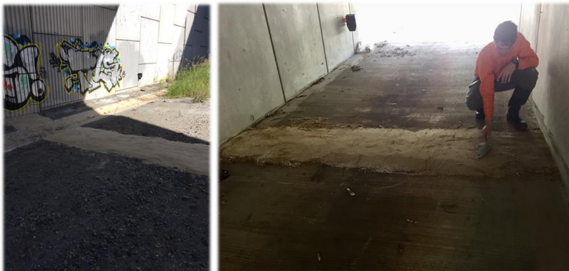
Plate 2: Underpass sand pad at Railway (L). Sand pad installation at Tyson's underpass (R).
