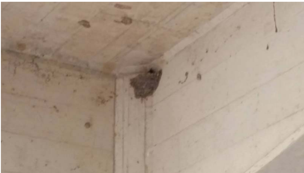
Plate 1-2. Micro bat suspected as Southern Myotis ( Myotis macropus ) inhabiting newly constructed swallow nests under the existing Pipers Creek Bridge.
