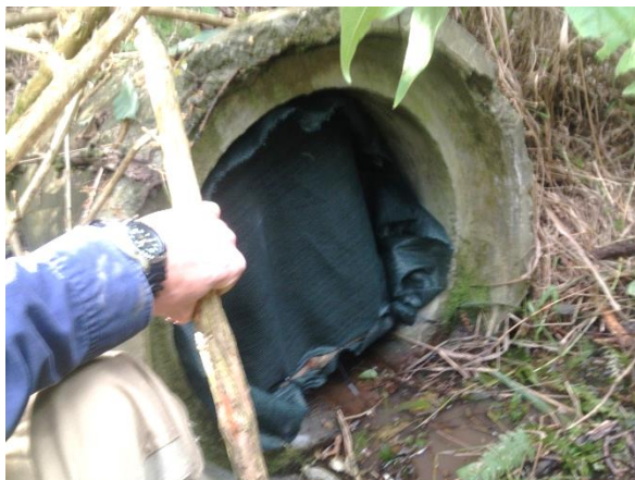
Plate 3. RCP 511067 (chainage 1000) was excluded with a nylon curtain after determining microbats were not roosting within the structure. The curtain features a 100mm gap at the base.
