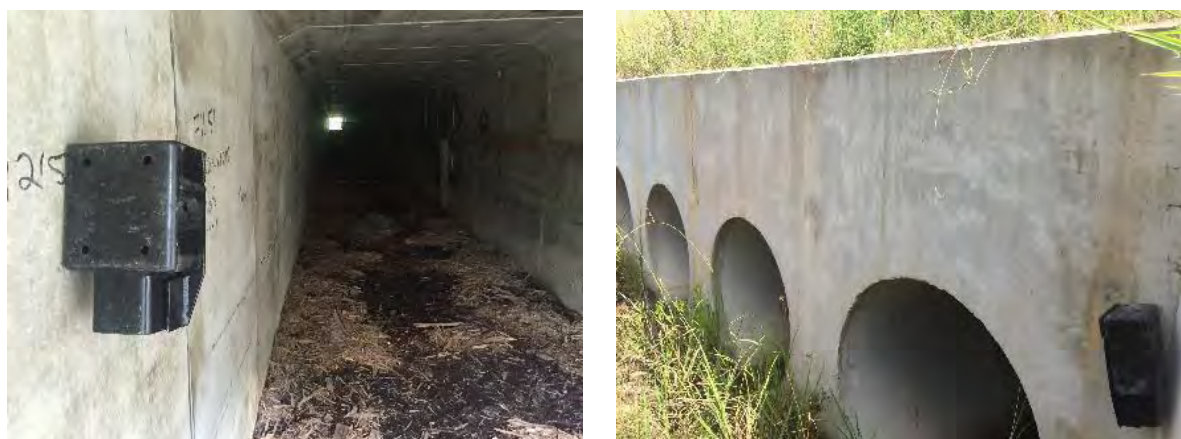
Plate 12: Single cell underpasses were monitored at each end with a Reconyx HC500 camera housed in a security case and mounted to the side wall opposite the wooden rail (e.g. Moonee underpass, left). For the pipe series at Emerald Beach, a camera was mounted on the wing wall at either side of the pipe series and directed across the entrance area on the east side (right).
