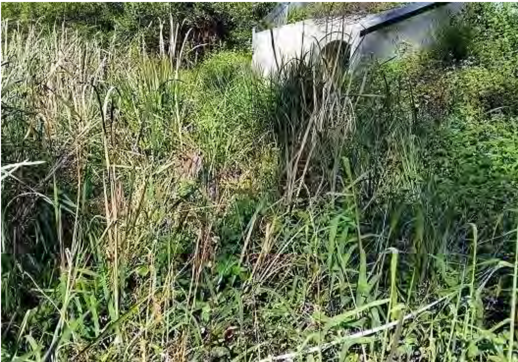
Plate 4: Habitat surrounding north-east frog pipe. The frog exclusion fence can be seen extending off the wing walls. (Picture taken 6 July 2017).
