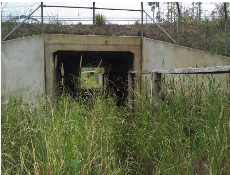
Plate 11: Arrawarra underpass north (ch.29930) viewed from the east (top), across the vegetated median (middle) and from west (bottom).
