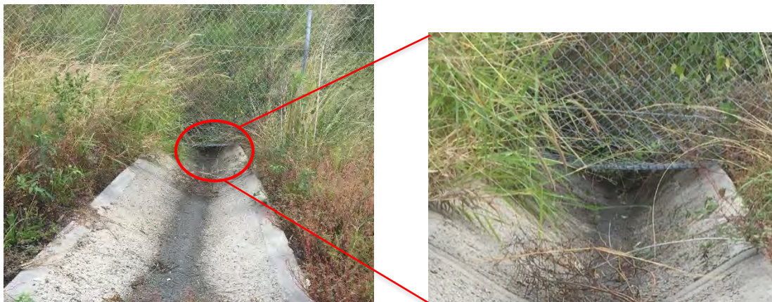
Plate 25: Concrete drains at a number of places along the Emerald west road mortality transect potentially compromise the fence integrity (bottom right).
