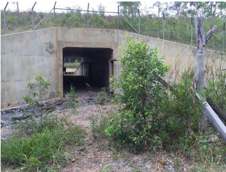
Plate 10: Arrawarra underpass south (ch.29380) viewed from the east (top), across the vegetated median (middle) and from west (bottom).
