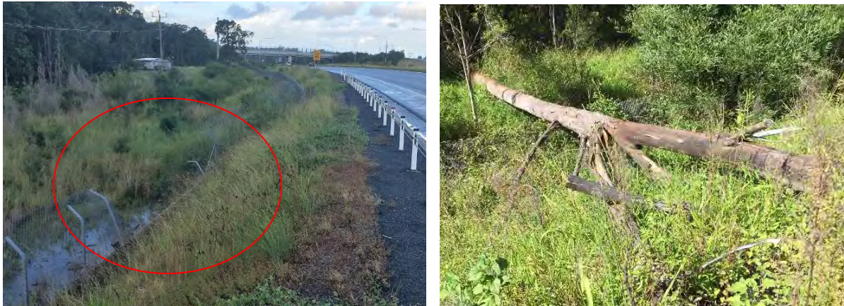
Plate 24: Breaches in the exclusion fence were evident at several locations including Emerald west where a vehicle had collided (top). A fallen tree potentially compromised the fence at vegetated median north east (bottom left).
