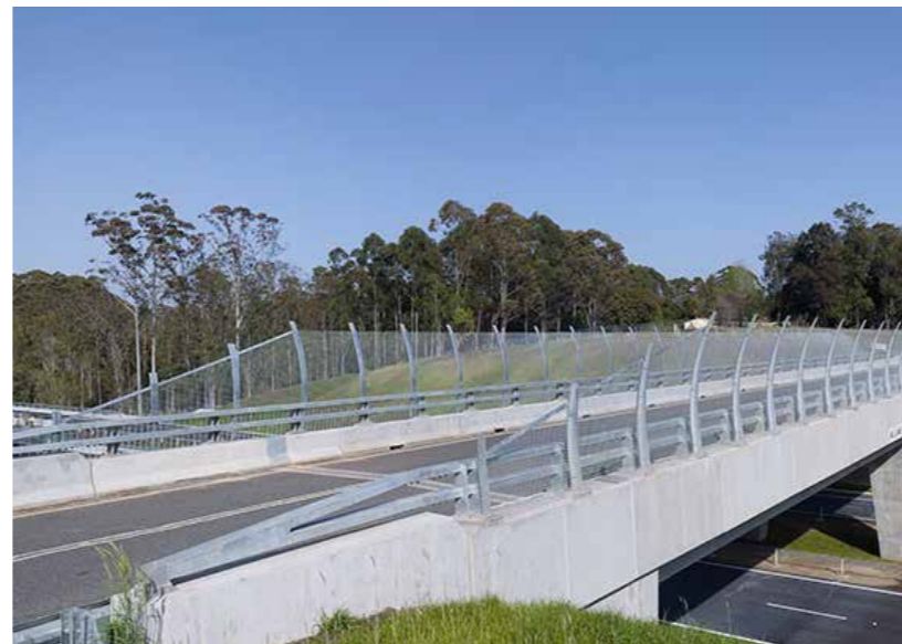
FIG A.7 EXAMPLE OF A THROW SCREEN ON A LOCAL ACCESS BRIDGE.
