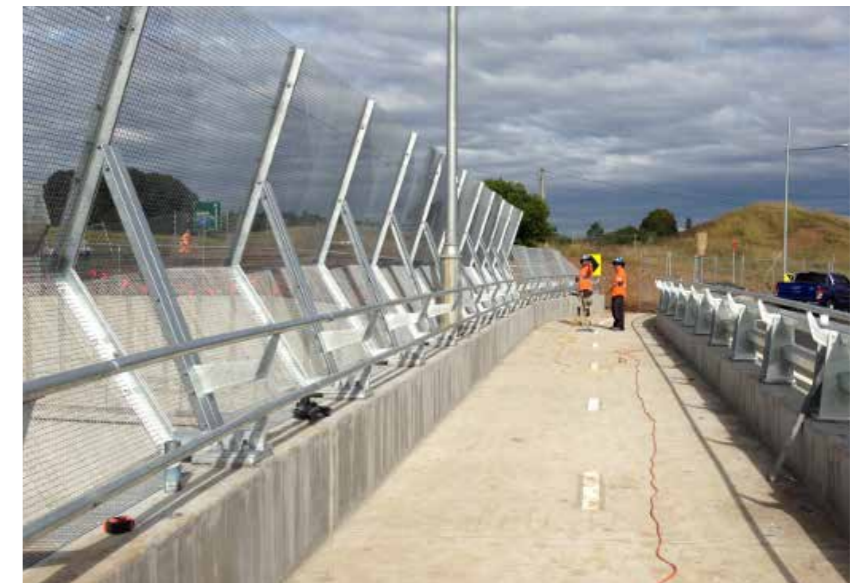
FIG A.8 A THROW SCREEN ADJACENT A BRIDGE WITH PEDESTRIAN FOOT TRAFFIC (BEING INSTALLED).
