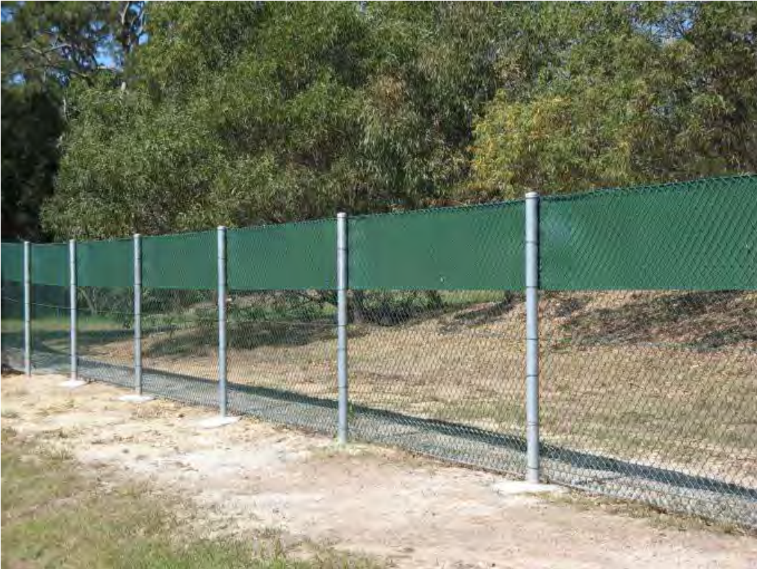
Figure 8 Koala exclusion fencing showing climbable materials with unclimbable metal sheet along the top (picture from EHP 2012)
