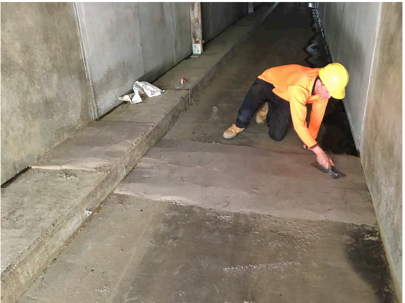
Plate 1: Sand pad being installed in a fauna underpass on the WC2NH upgrade.
