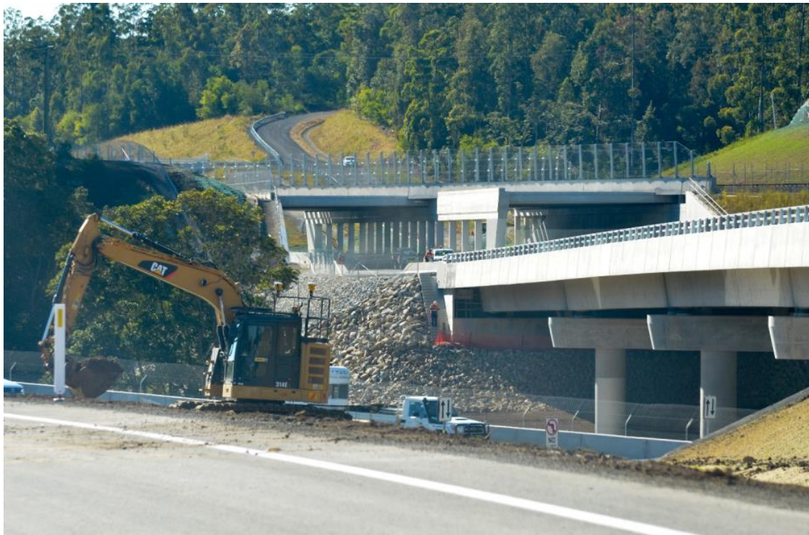
Photo 2: South Western view of Warrell Creek Bridge with the Pergola in the background
