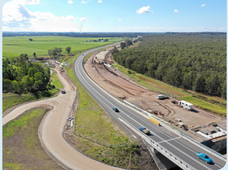
Almost four kilometres of new single carriageway open to two-way traffic between Maclean and Yamba
