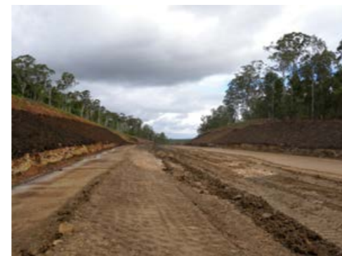
Figure F8: Glenugie upgrade April 2011.
