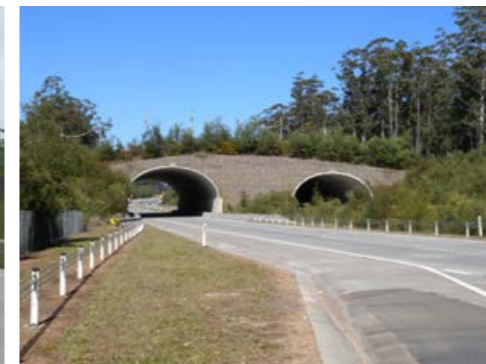
Figure F5: Bonville Koala Bridge September 2011.
