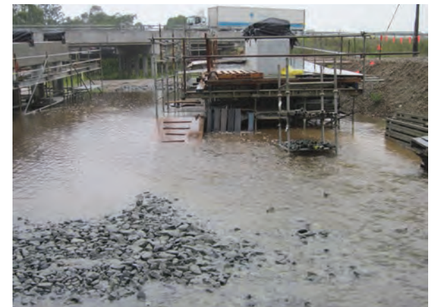
Heavy rain on the Herons Creek to Stills Road upgrade (January 2012)
