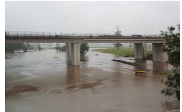
Heavy rain on the Bulahdelah upgrade (January 2012)
