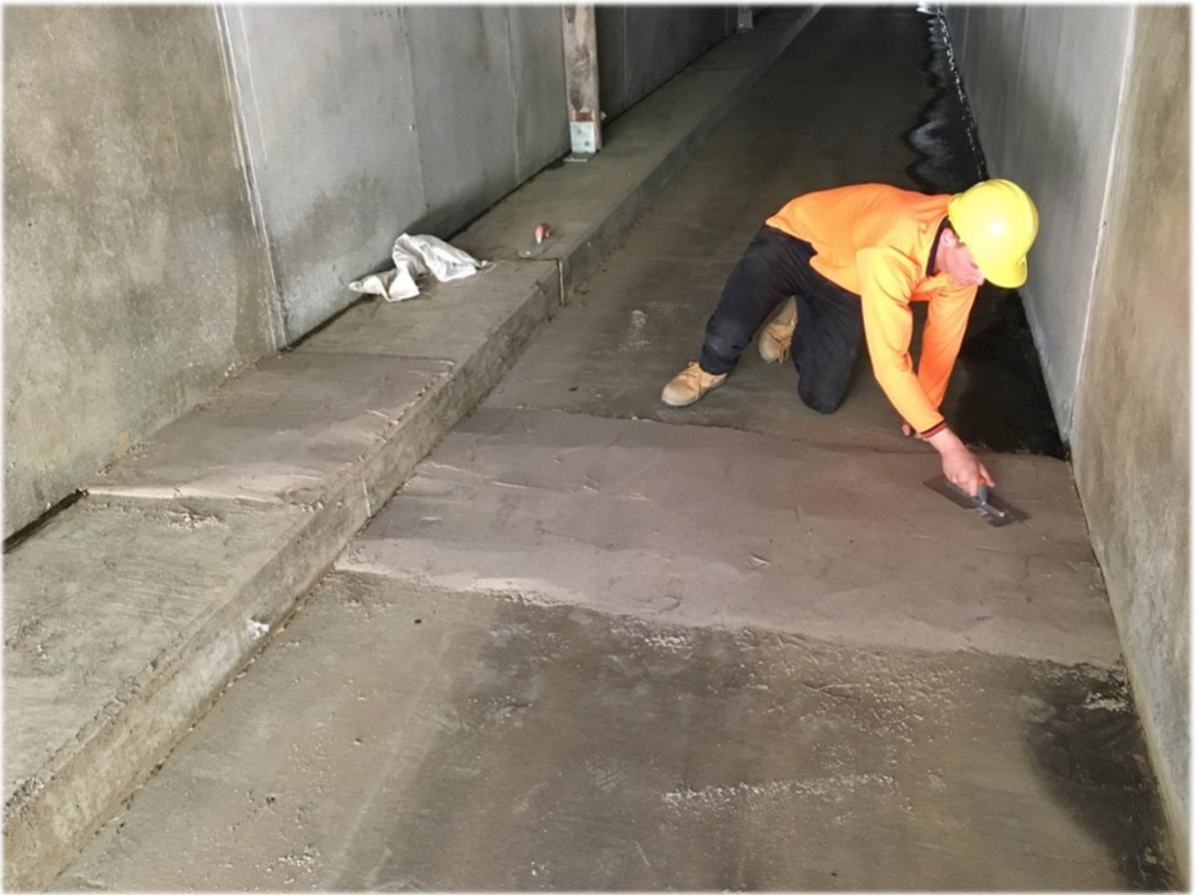
Plate 2: Sand pad being installed in a fauna underpass on the WC2NH upgrade.
