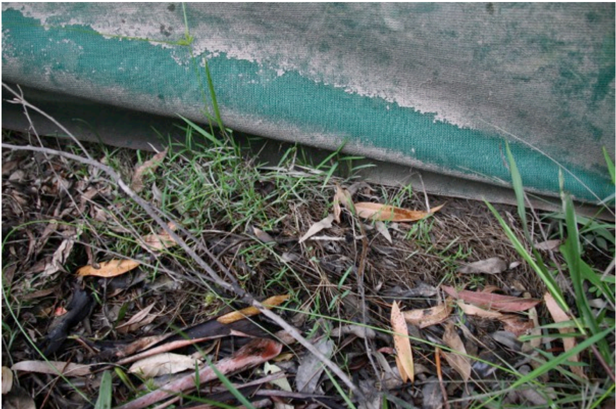
Plate 13. Floyds Grass Receival Site 9, Area 2. There is still a reasonable amount of Floyds Grass growing amongst Broad-leaved Paspalum which would have a much better chance of survival if the site had more maintenance, which it missed out on during the construction period.
