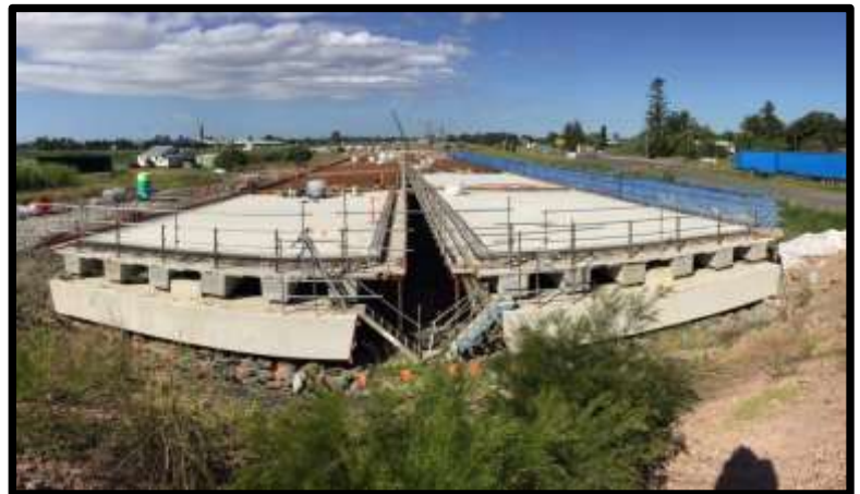
Constructing the bridge deck at Bridge 52 North of Watts Lane, Harwood Island, April 2018. Bridge 52 will be 380 metres in length when completed.
