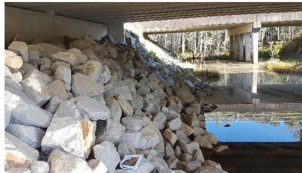
Plate 4.4 Southern bank at SBT2 with rock scour protection and no obvious path that crossing fauna need to navigate.
