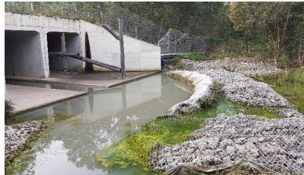
Plate 4.2 Scouring and pooled water at the outlet of C8.
