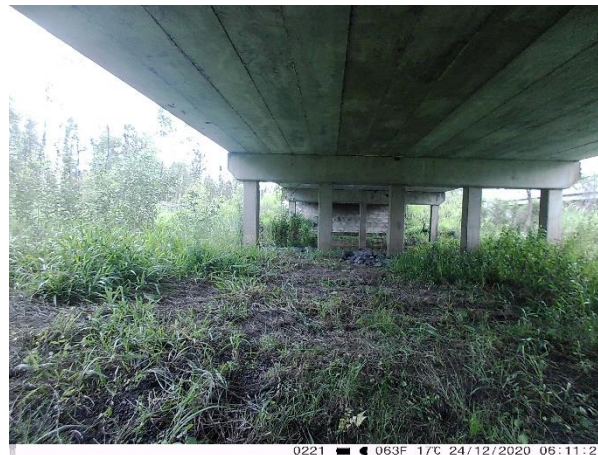
Plate 4.6 Southern bank at NBT3. The vegetation has been trimmed in this photo to prevent obstruction of camera traps. The image shows that the passage for crossing fauna consists of regular flat ground.
