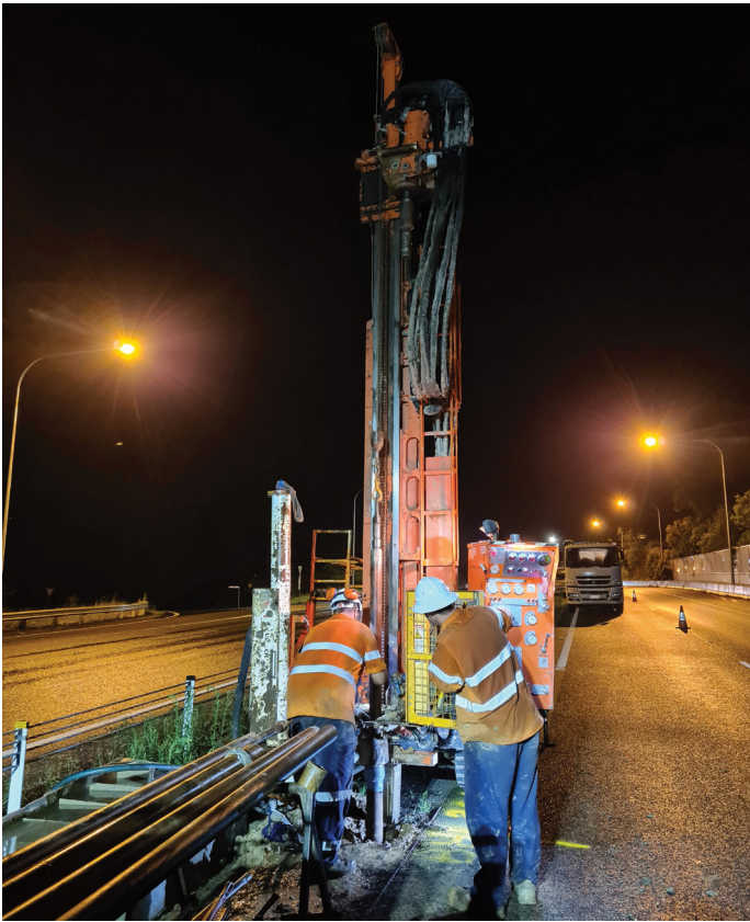
Geotechnical investigations at night along the Pacific Highway, Korora to Sapphire Beach
