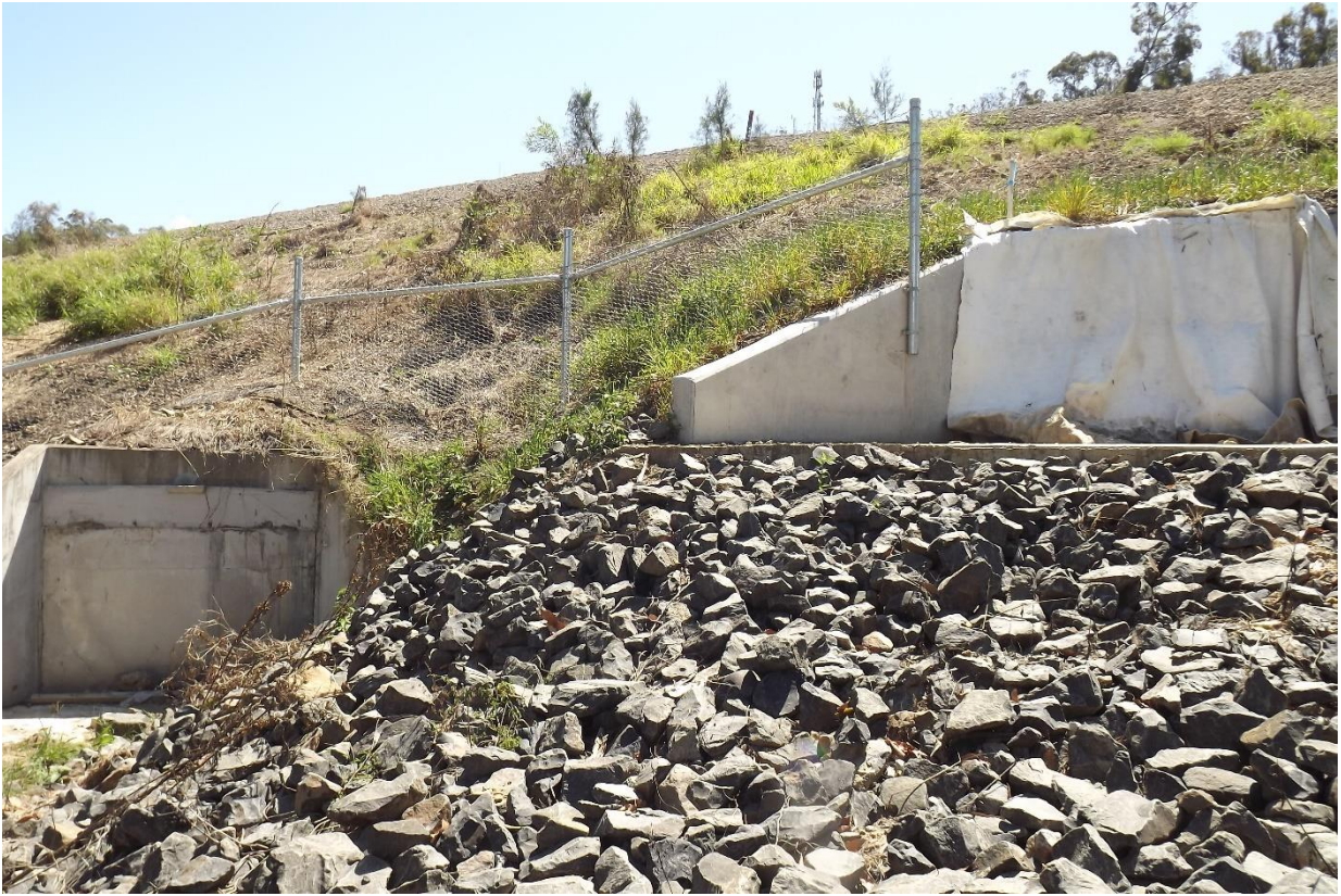
Plate 15: Original box culvert (now sealed, lower LHS) and newly constructed culvert (upper, RHS) at Maclean cut, October 2019.
