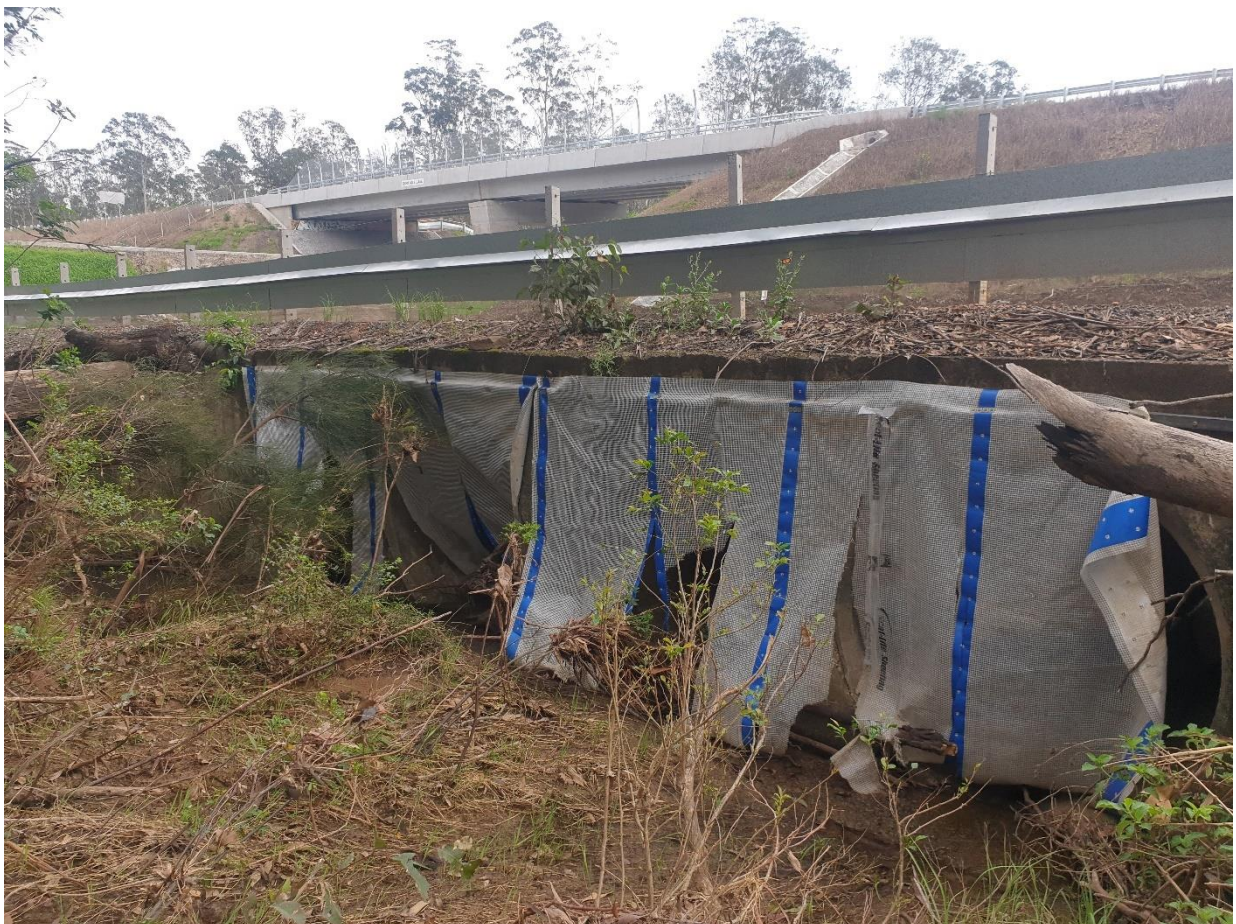
Plate 11: The original Picaninny Creek culvert showing exclusions still semi-intact following flooding in January 2020.
