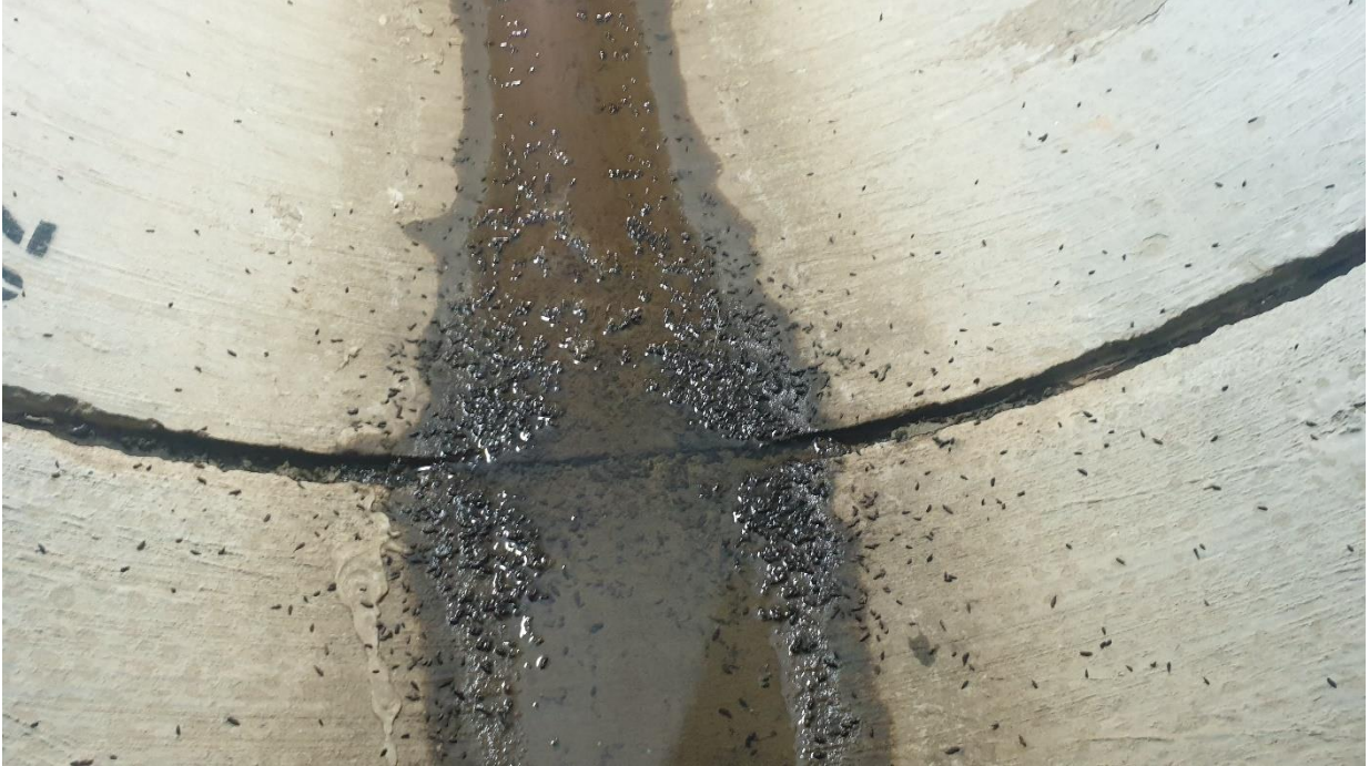
Plate 14: Microbat guano beneath an expansion joint of one of the new Maclean cut culverts, August 2020.
