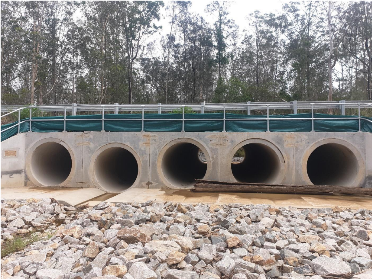
Plate 12: Newly installed culverts at Pheasants Creek, Eight Mile Lane, Glenugie Link, Section 3A, October 2019.
