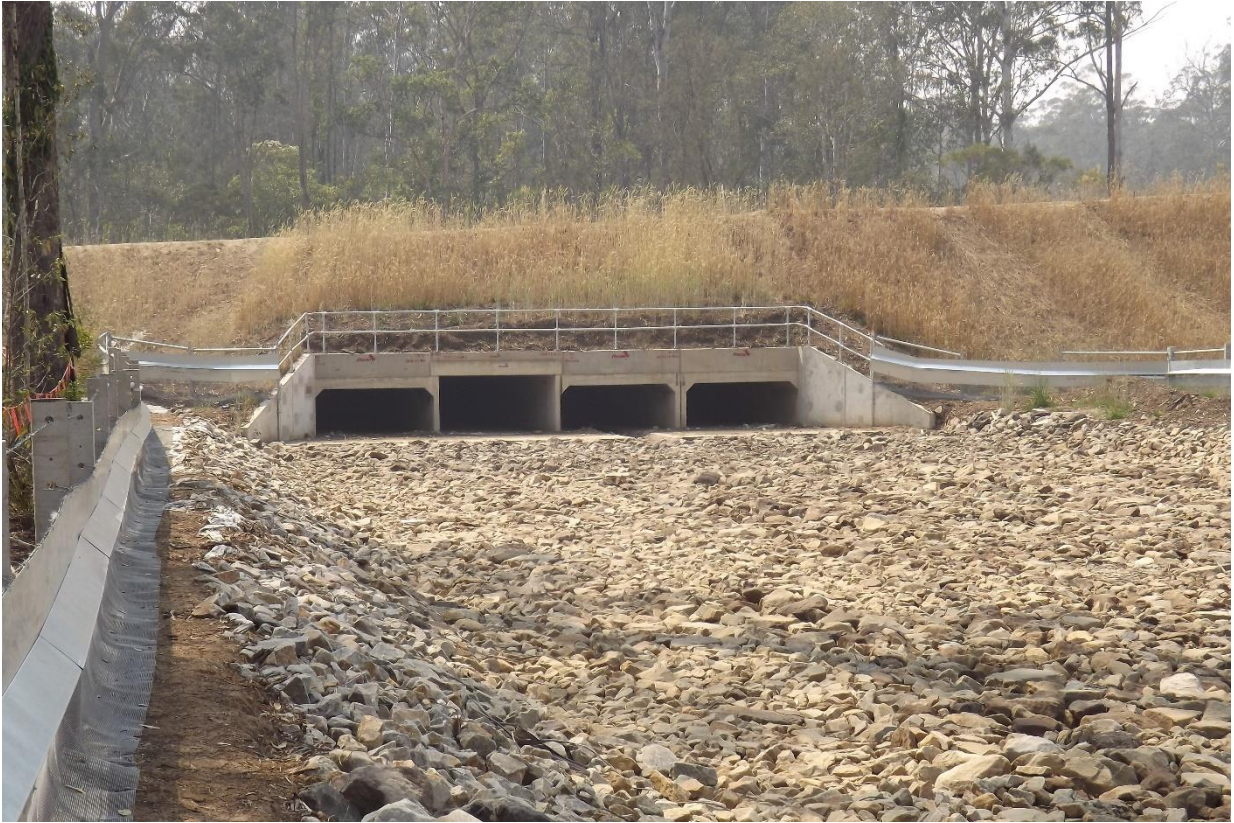
Plate 13: Newly installed culverts at Picaninny Creek, Eight Mile Lane, Glenugie Link, Section 3A, October 2019.
