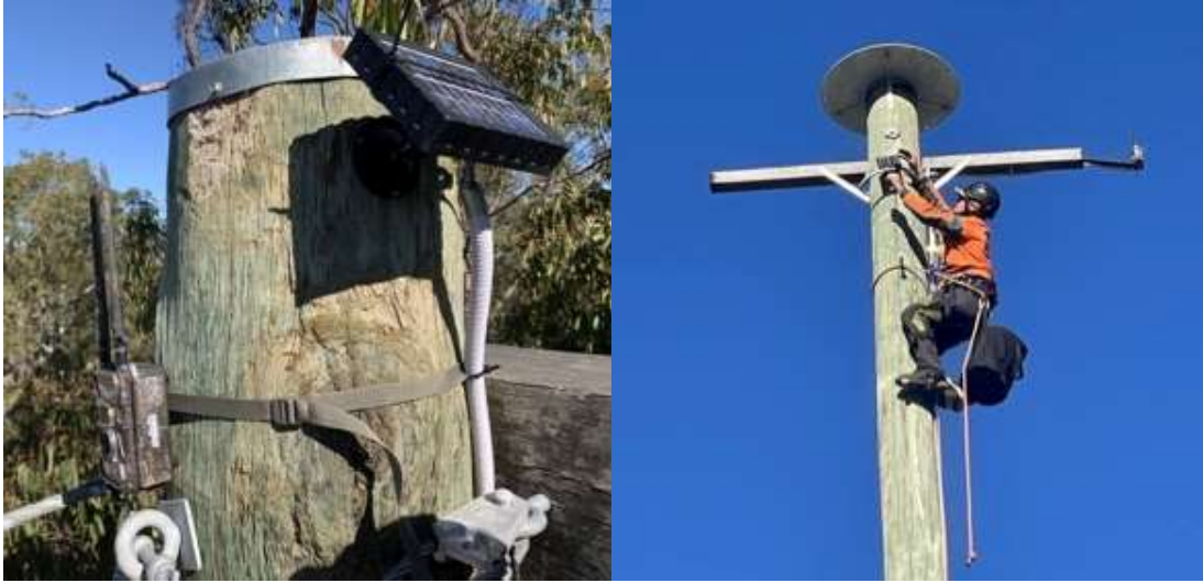
Plate 2: Location of camera attachment on rope bridges (left) and glide poles (right) in S3-11. Each structure contained a wireless 4G Enduro camera with a small solar panel.
