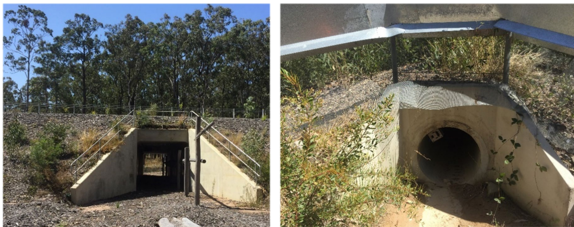
Plate 1: The majority of monitored box culverts contained timber post-and-rail furniture and some featured mulch spread over the concrete floor (left). Pipes did not feature fauna furniture or mulch (right).
