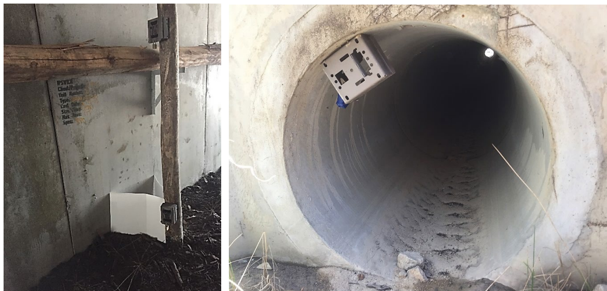
Plate 2: Cameras were installed on the centre post within each box culvert – one viewing along the rail and the other along the floor (left). White core-flute sheeting was placed between the side wall and the post to direct fauna past the camera.
