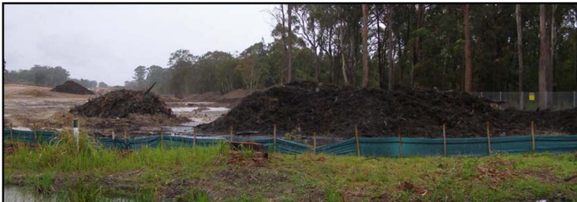
Plate 6: Mulched vegetation stockpiled in a low-lying area subject to inundation. This is not an appropriate stockpile location and may increase the generation of tannins from stockpiled mulch.
