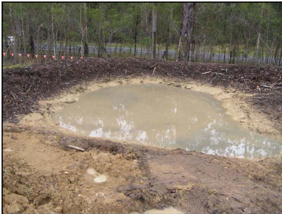
Plate 12: Mulch used as a bund for a temporary sedimentation catch dam. Mulch is effective as it can provide both containment and filtering of site water. Mulch should not be used as a control in areas of concentrated flow where it may be washed away. Any mulch containment control should have a defined and lined outlet that allows discharge from the control without washing mulch away. Note that this control does not have a defined discharge outlet which should be installed to prevent failure of the control in heavy rainfall events.
