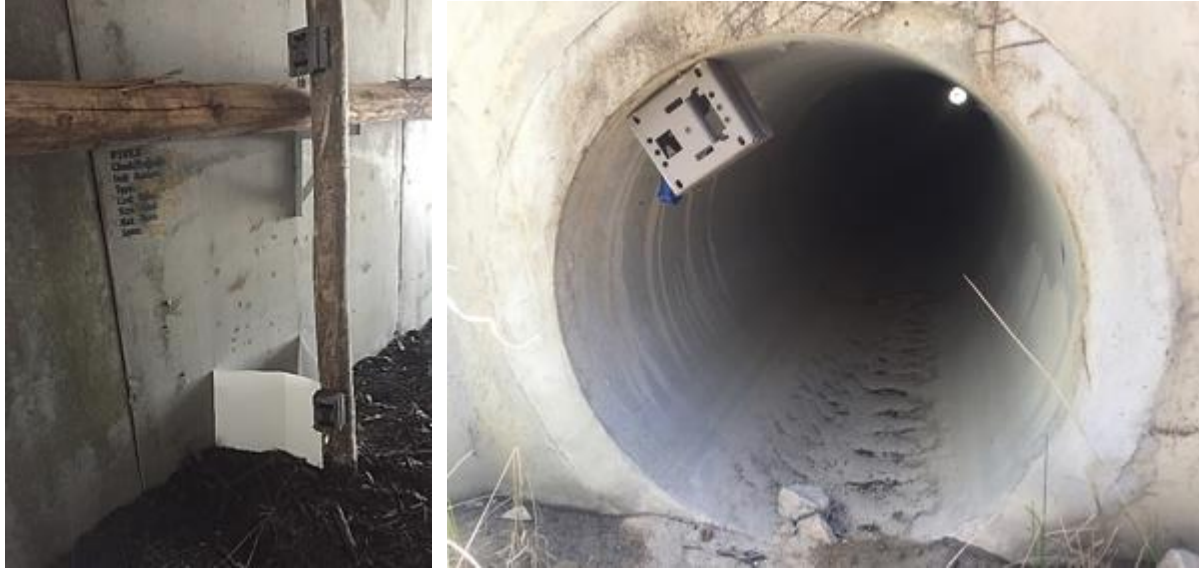
Plate 2: Within each box culvert, cameras were installed on the centre post— one viewing along the rail and the other along the floor (left). Within pipes, cameras were installed on the upper edge of the obvert (to reduce inundation) and angled towards the floor.
