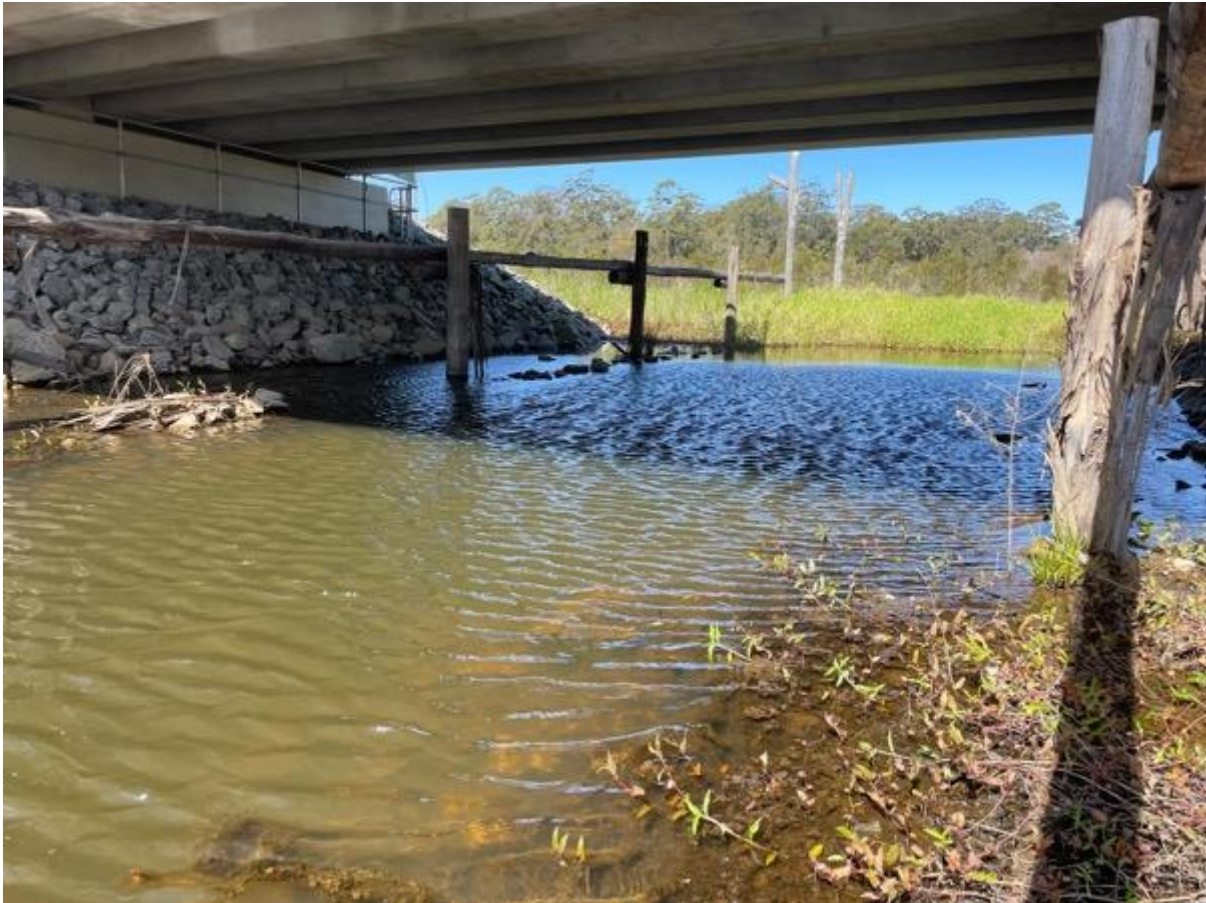
Plate 1: Bridge underpass (M68/K54) remained inundated throughout 2022. This photograph was taken in August 2022 six months after the initial flood event.
