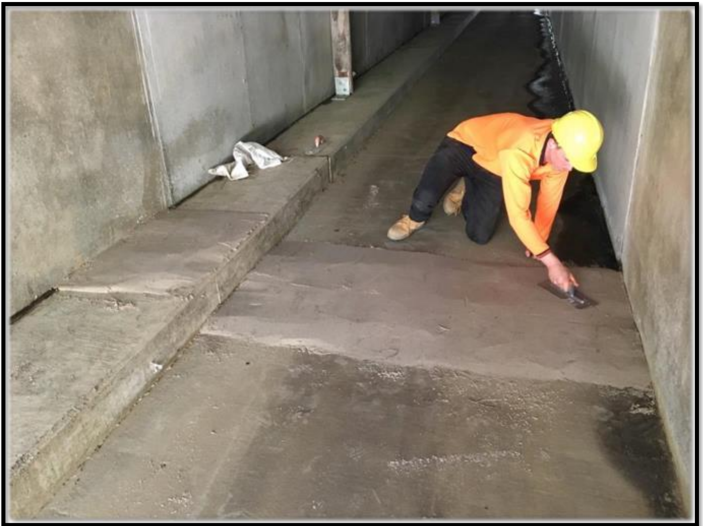
Plate 2. Sand pad being installed in a fauna underpass (Site 3) on the WC2NH upgrade.
