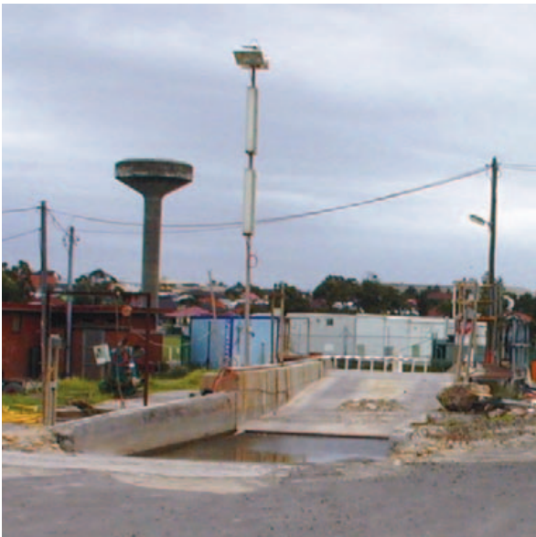
FIGURE 7.7: Wheel wash bay used at Tempe Reserve during construction of the Airport Link, Sydney Region. Most trucks drove through the wheel wash, but some vehicles needed to be scrubbed to ensure materials were not transported from site. The water depth was approximately 400mm, with a cattle grate underwater for solids to settle under (Photo: Leigh Trevitt).
