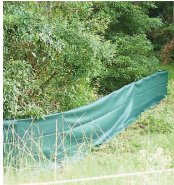
FIGURE 9.8: Temporary frog fencing installed for the Sapphire to Woolgoolga project to prevent the endangered Giant Barred Frog ( Mixophyes iteratus ) from entering construction areas (Photo: Josie Stokes).
