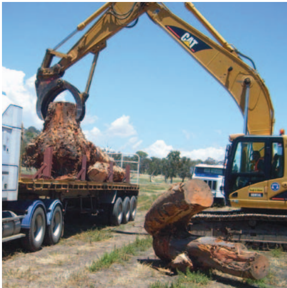
FIGURE 5.4: The RTA provided trees felled for the Hume Highway duplication project for the Murray River Resnagging project. Large logs were transported by truck from the road works site (Photo: M Casey, DPI).
