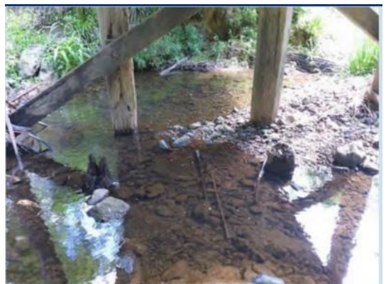
Photograph 4 Remains of previous bridge
