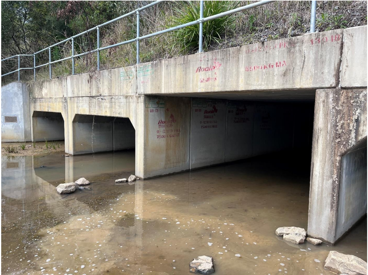
Plate 6: Newly constructed Picaninny Creek four cell culvert (CH 35880), Eight Mile Lane, Glenugie Link, Section 3A
