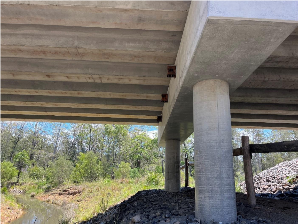
Plate 7: Three x four chambered bat boxes installed beneath the new Pheasants Creek Bridge, February 2023
