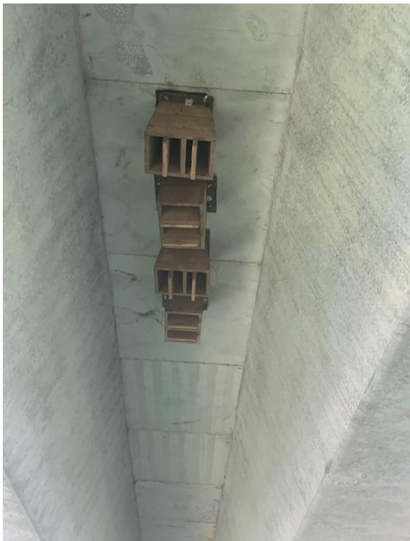
Plate 12: Four additional timbered four-chambered microbat boxes beneath Mororo Bridge (October 2023).
