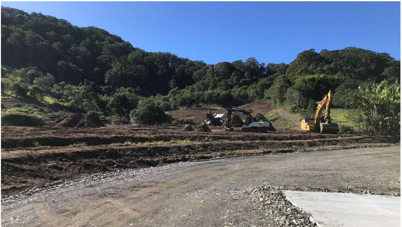
Photo 4 – Clearing and ground preparation work being undertaken at the Mackeys Rd worksite
