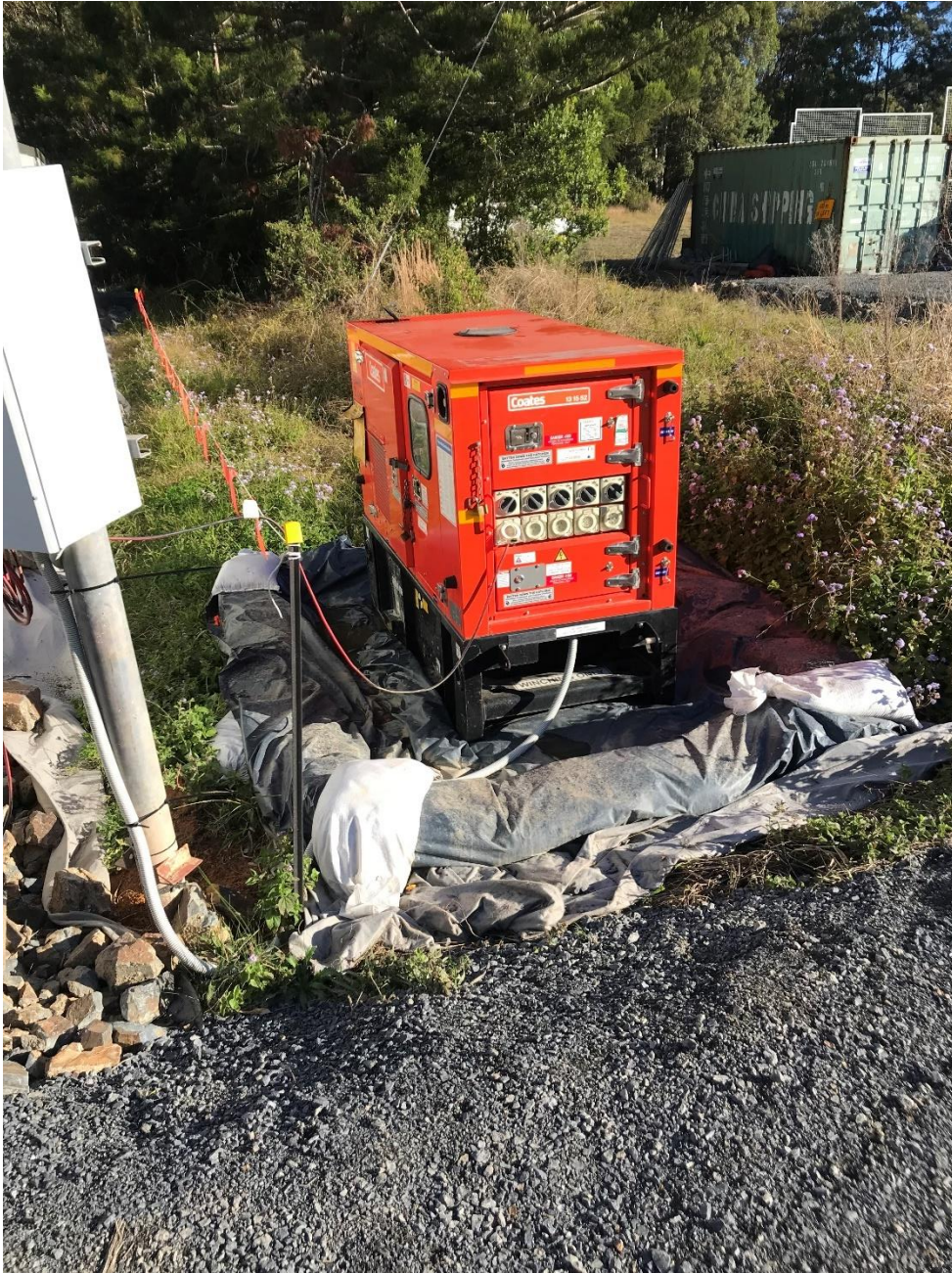
Photo 13 – Self bunded generator placed within another bund at Satellite compound IJ
