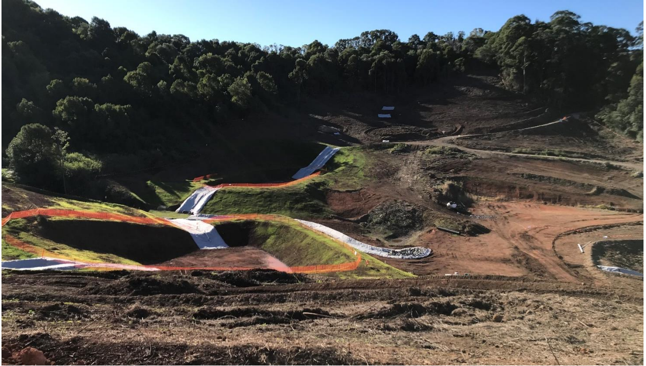
Photo 9 – Sediment basin and water diversions at Earthworks at Cut 4, Fill 3D worksite
