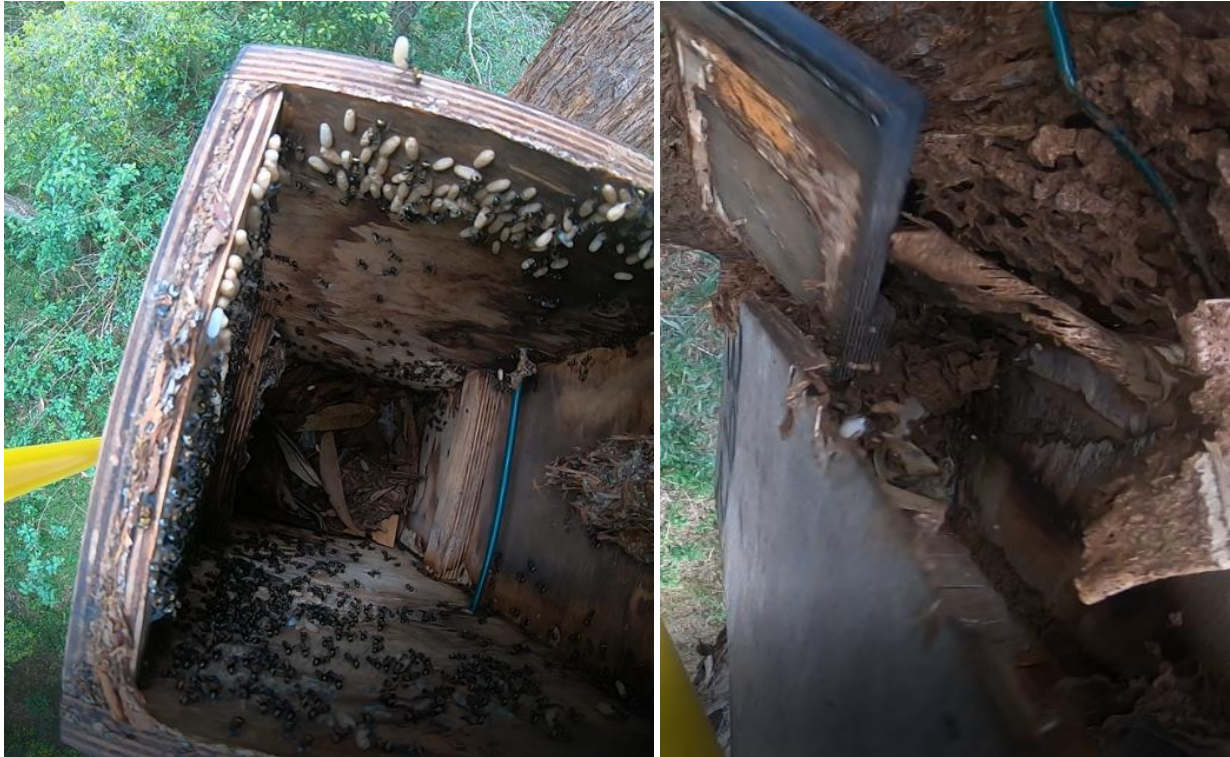
Photo 10: left: Timber box infested with ants, Spring 2021. Right: Timber box infested with termites, Spring 2021.
