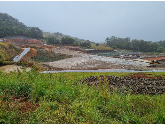
Image 7: Fill 14, Gatelys Rd tunnel south portal (Ch20000 - 20400) – Site during 27/10 rain event
