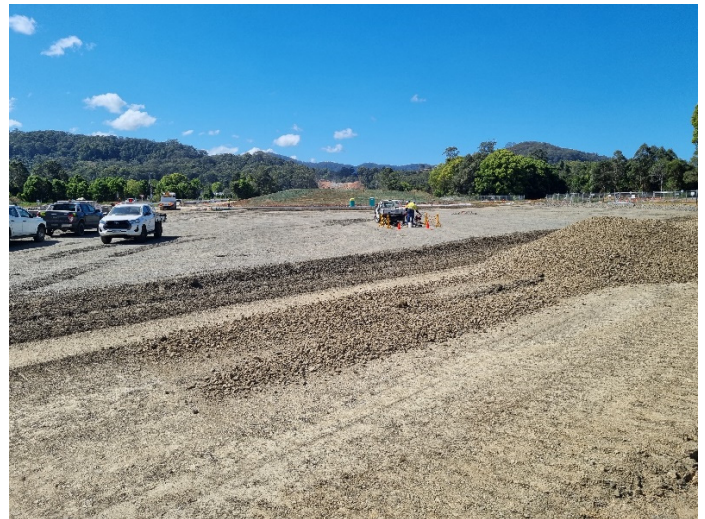
Image 4: North Boambee Rd, looking north to Fill 3D (Ch12000 - 12600) – Earthworks and piling pad construction
