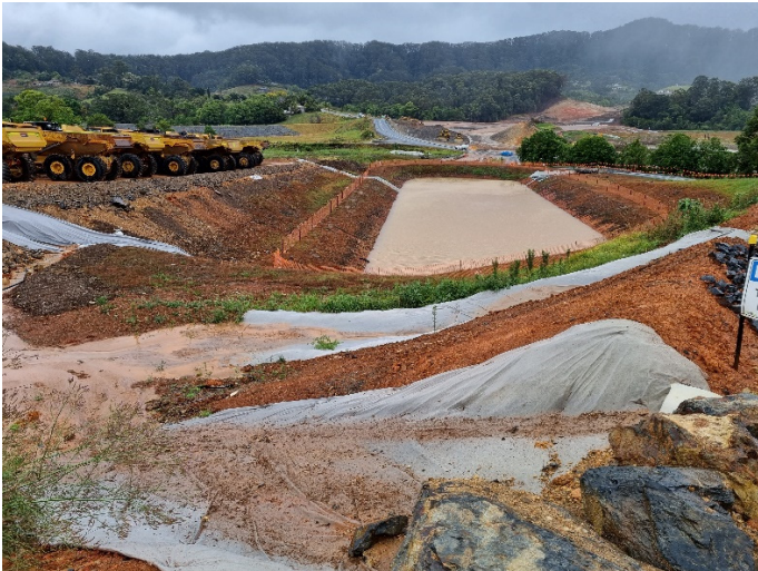
Image 5: Fill 6A, south of Coramba Rd (Ch14400 - 14700) – Runoff into sediment basin during 27/10 rain event
