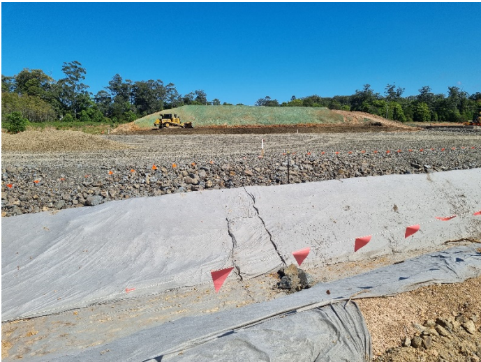
Image 3: Bridge 23, south of Nth Boambee Rd (Ch12000) – Piling pad in preparation for bored piling
