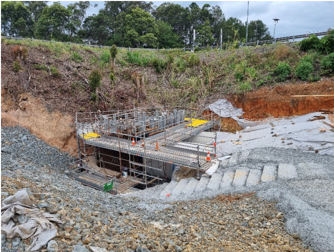
Image 5: Bruxner Park Rd / Pac Hwy intersection (Ch20800) – Construction of major stormwater drainage pit
