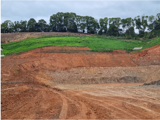
Image 1: Roberts Hill tunnel north portal (Ch13700) – Earthworks at tunnel entrance and hydromulch above
