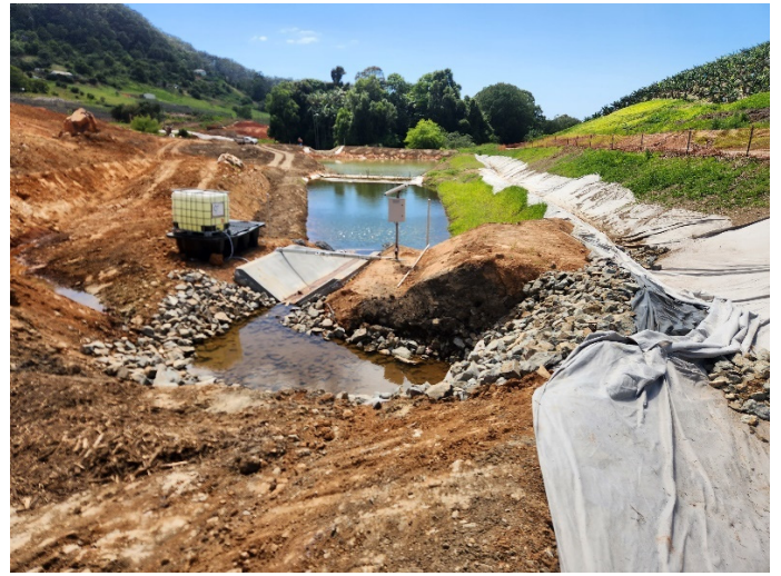
Image 6: Shephards Ln tunnel north portal (Ch17500) – Sediment basin and adjacent clean water diversion drain
