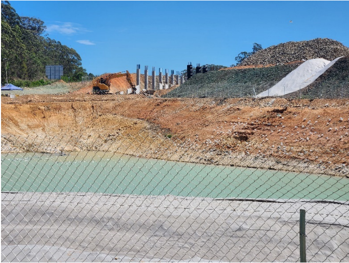
Image 1: Englands Rd Interchange, south side (Ch10700) – Sediment basin, with bridge piles in background
