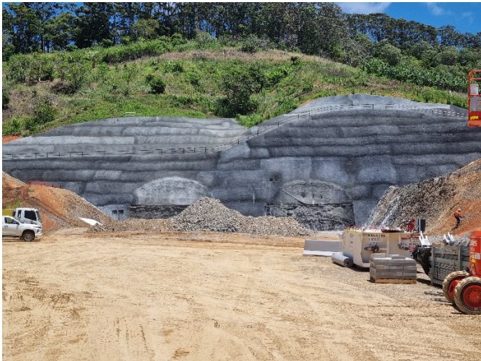
Image 7: Gatelys Rd tunnel north portal (Ch19300) – Preparation of portal for commencement of tunnelling works
