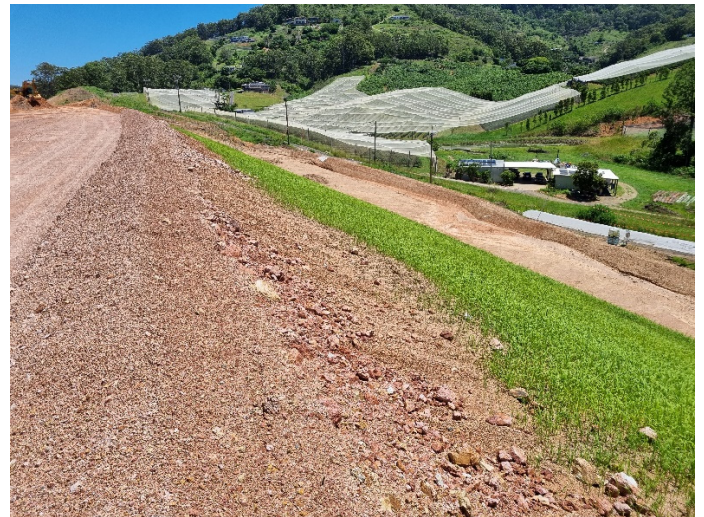
Image 8: Korora Hill, Fill 18 (Ch21700) – Fill batter that has been recently hydromulched with permanent seed mix
