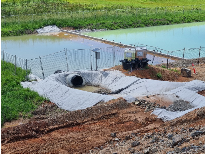
Image 5: Coramba Rd, north side, Fill 7 (Ch15200) – High efficiency sediment basin following rainfall
