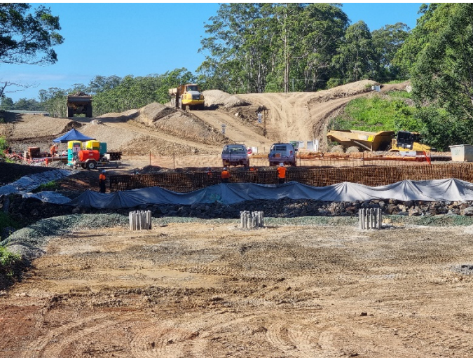
Image 3: North Boambee Rd, south side, Bridge 3 (Ch11700) – Piling complete, preparation for headstocks underway
