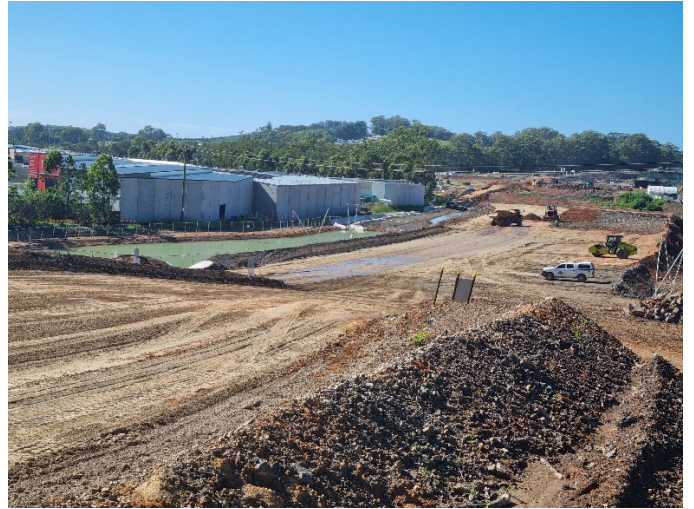
Image 2: Englands Rd, Fill 2B (Ch11500) – Looking south with sediment basin on left, adjacent to industrial area
