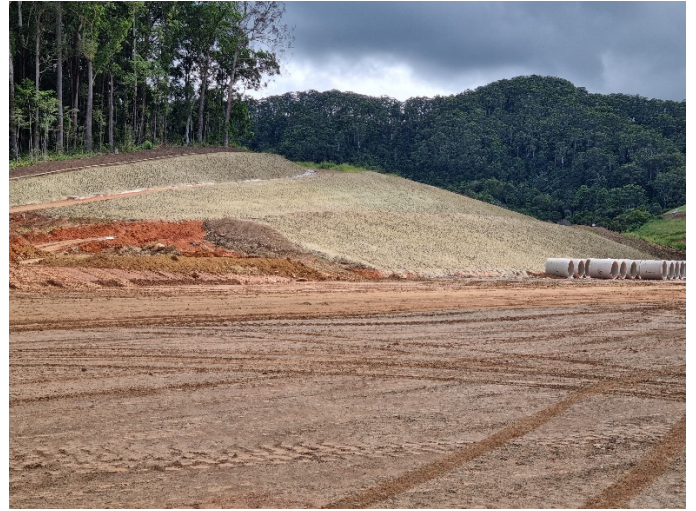
Image 2: Coramba Rd (nth side), Cut 8 (Ch15400) – Western batter that has been recently hydromulched
