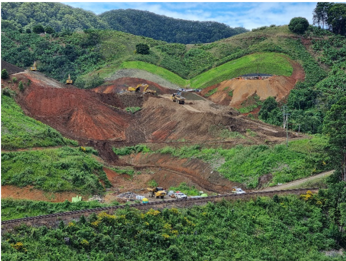
Image 3: Shephards Ln tunnel south portal (Ch17000) – Looking across railway line towards earthworks at portal
