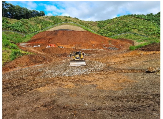
Image 4: Shephards Ln tunnel north portal (Ch17300) – Earthworks and shotcreting at tunnel portal
