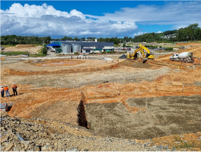
Image 1: Englands Rd, Fill 2B (Ch10900) – Looking east across future interchange roundabout to Isles Drive
