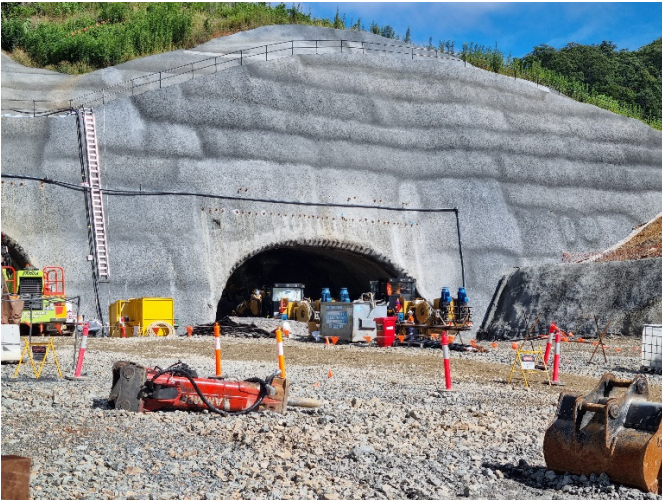
Image 5: Gatelys Rd tunnel north portal (Ch19300) – Initial tunnelling works, including rock hammering and drill & blast
