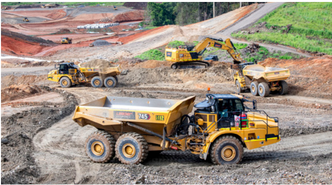
Excavators loading dump trucks at Coramba Road interchange with rollers in action in the background
