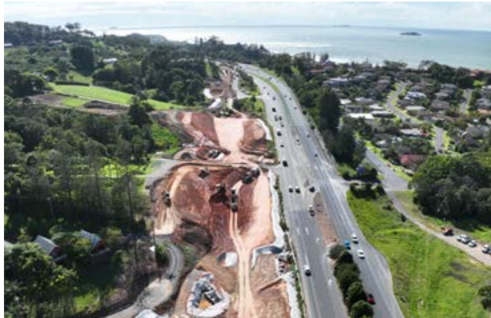
The northern tie-in of the Coffs Harbour bypass with the Pacific Highway near Korora, pictured (top) in February 2024 and (bottom) in April 2024.
