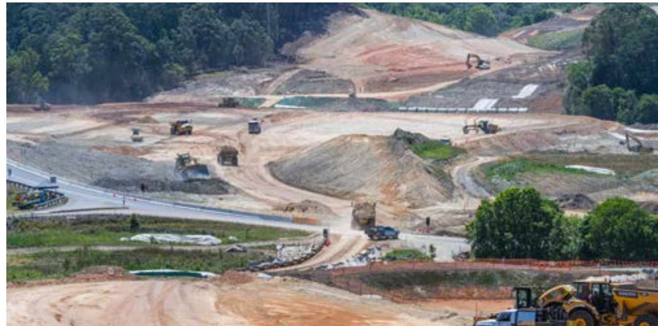
Above: works just north of Coramba Road pictured (top) in September and (below) October 2023.
