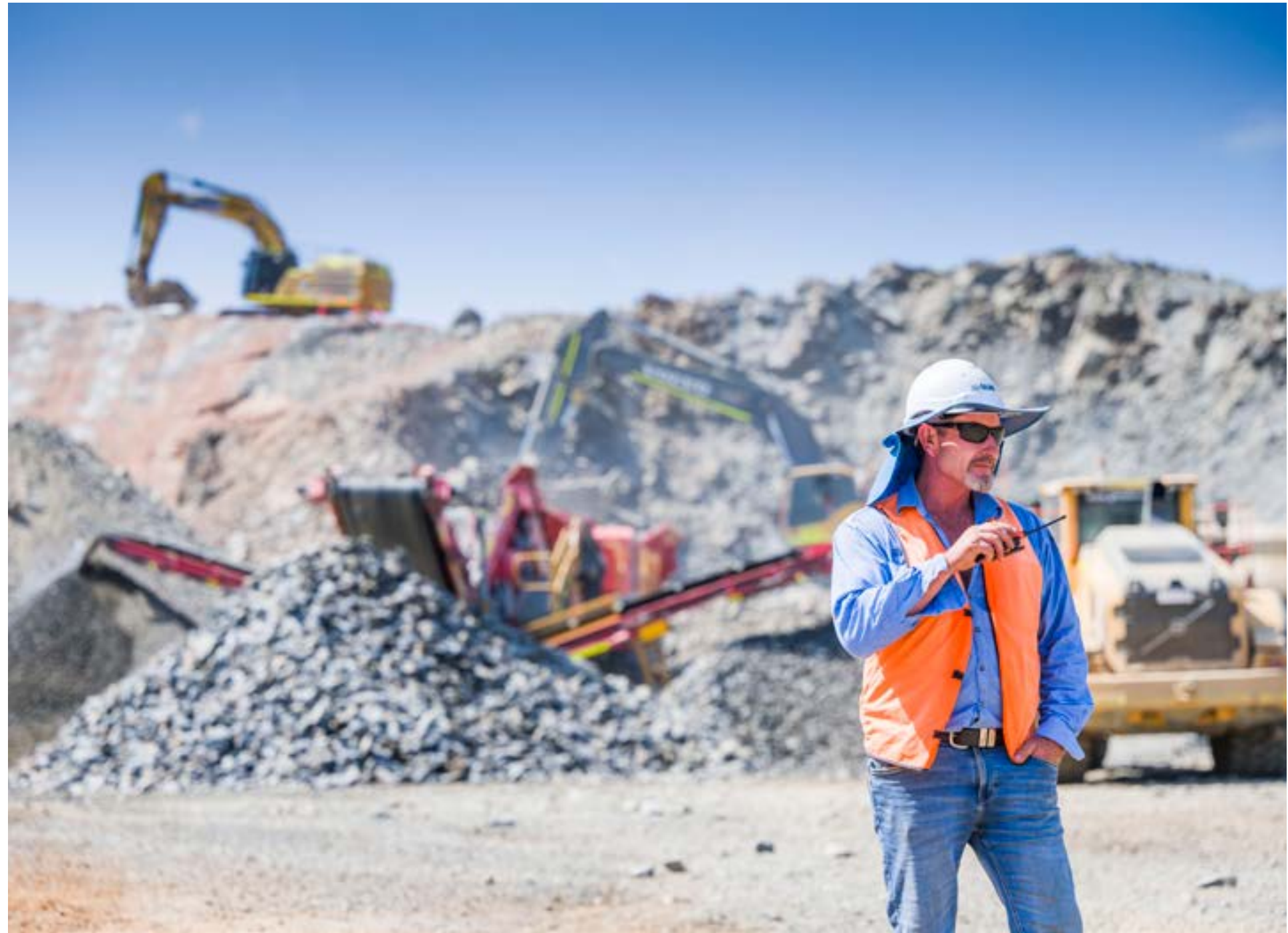
Construction senior supervisor coordinates plant in the southern area of the bypass.
