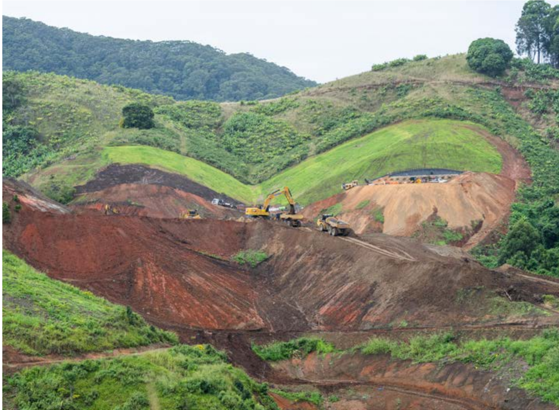
Shephards Lane Tunnel southern portal takes shape with tracks and benches cut into the hillside.
