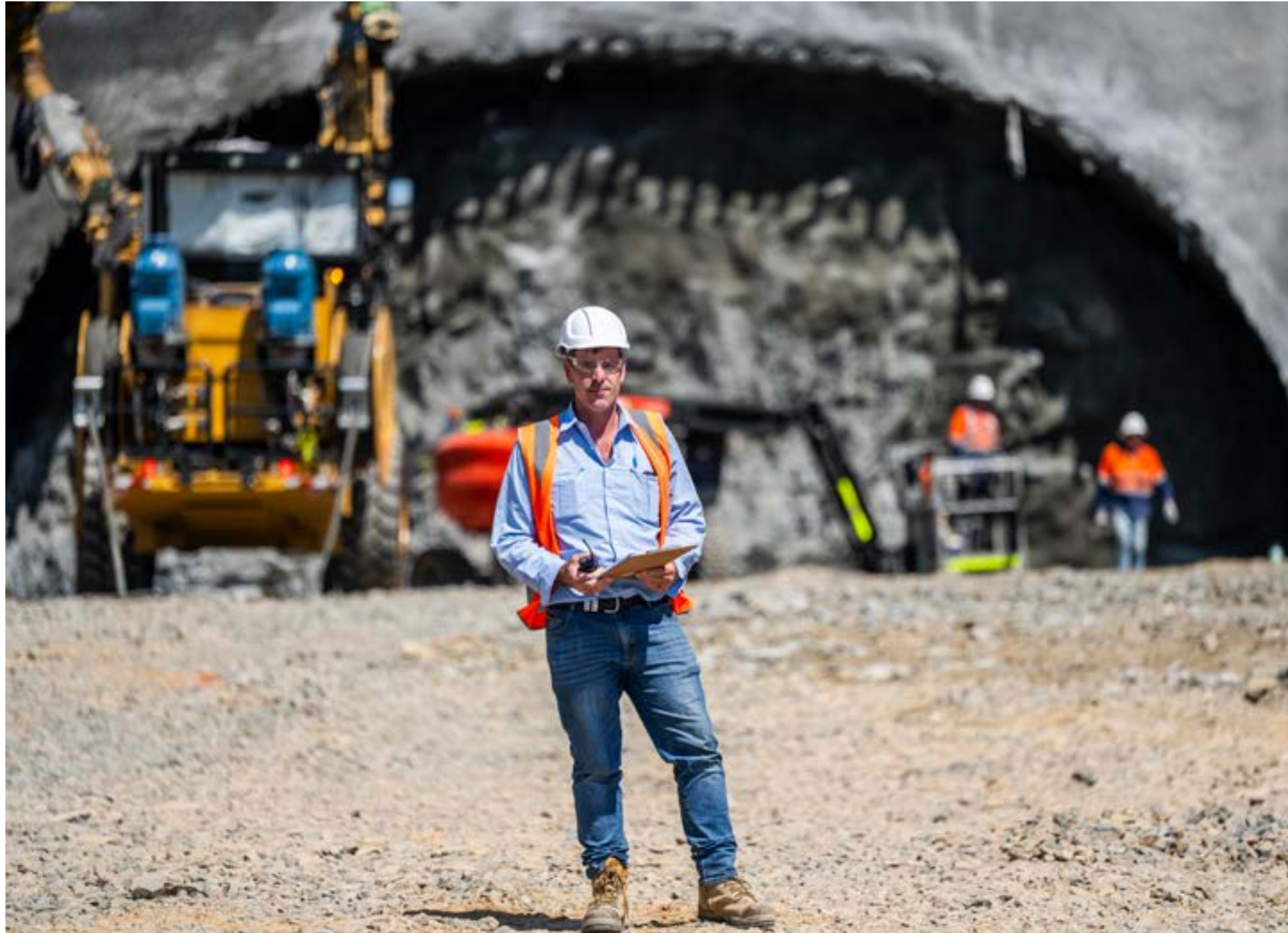
A superintendent oversees controlled blasting of the tunnel tubes at Gatelys Road, pictured in late February 2024.
