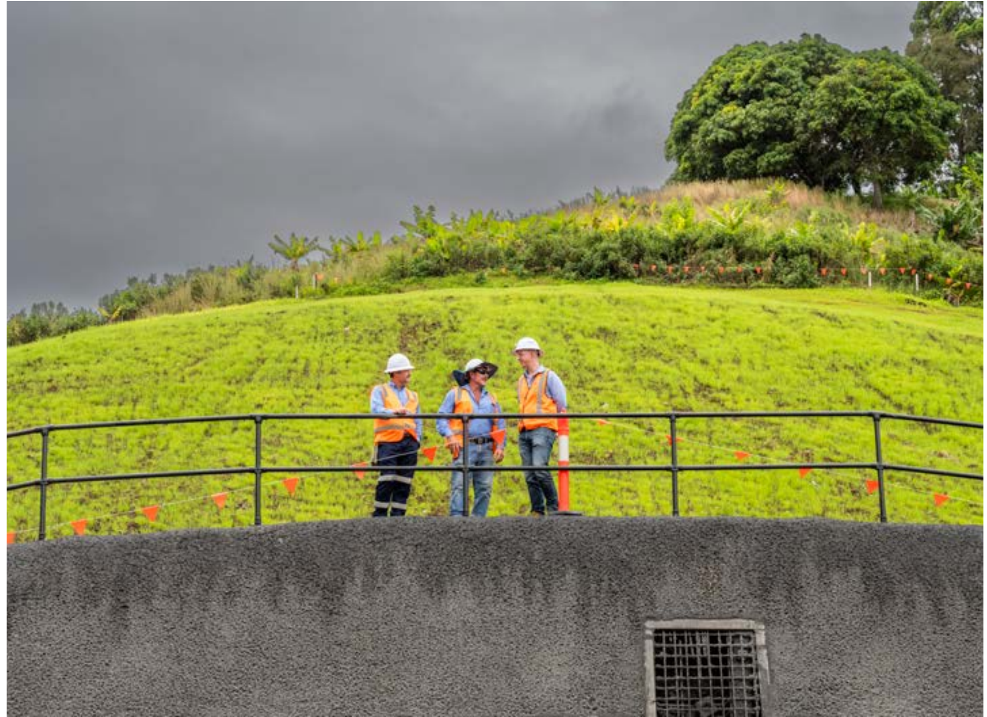
Construction senior supervisor and project managers from Transport for NSW and Ferrovial Gamuda Joint Venture meet at the top of Shephards Lane Tunnel.
