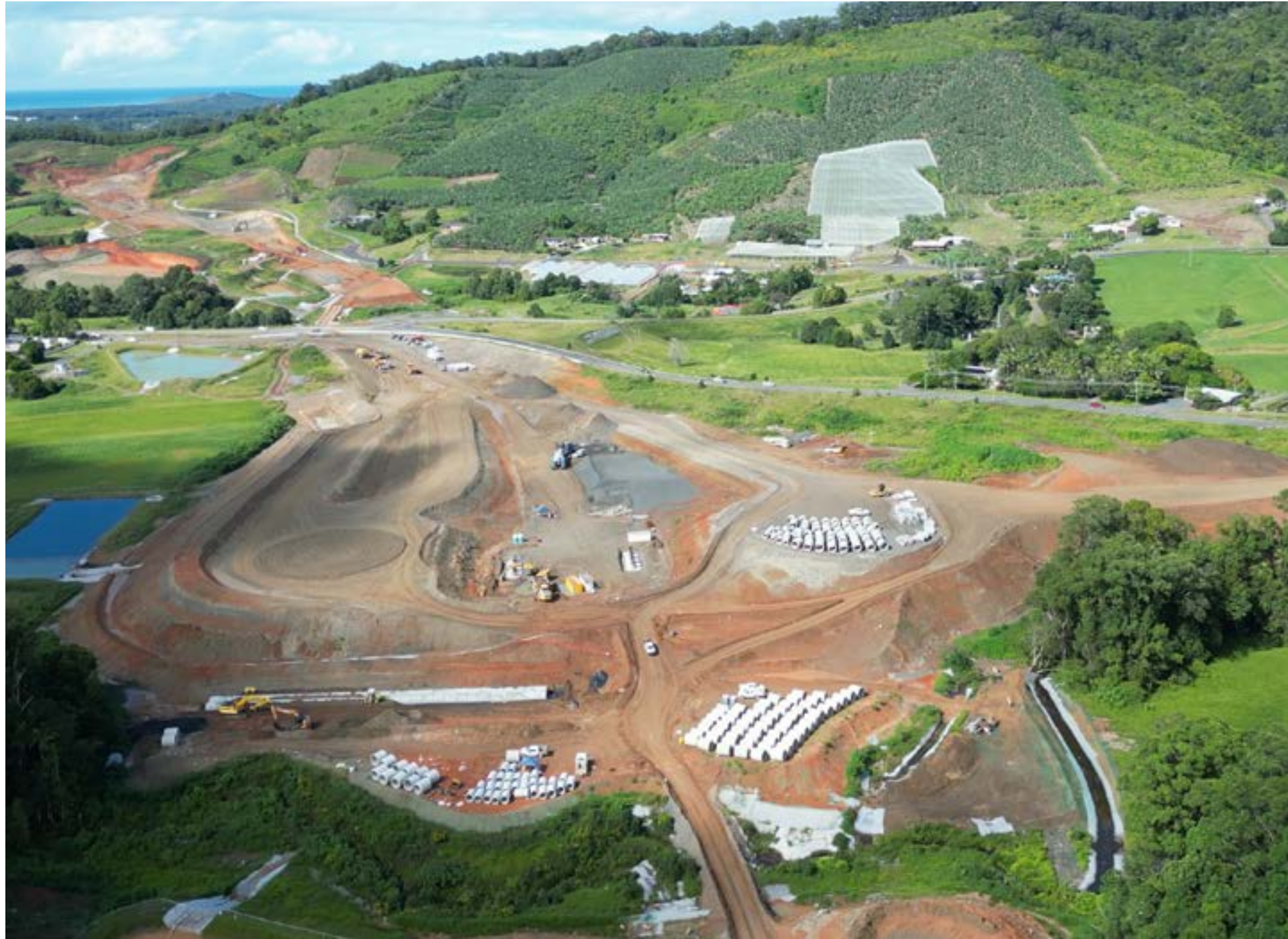
Aerial view of construction of the Coramba Road Interchange, looking south towards Roberts Hill.
