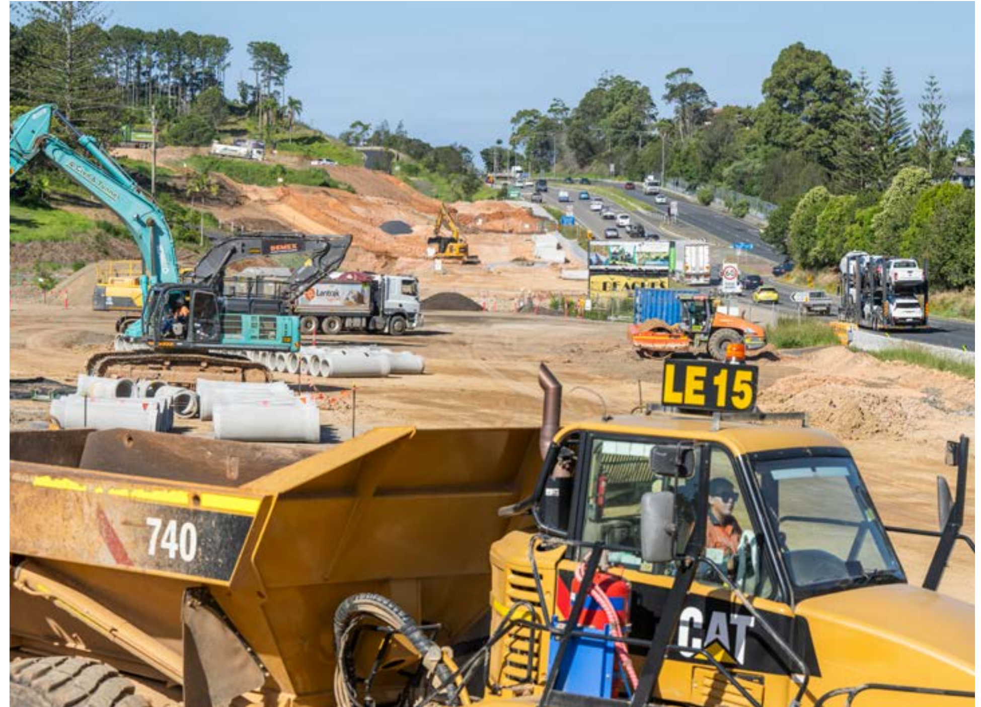
Plant operators working hard to progress the northern section of the Coffs Harbour bypass, pictured in January 2024.
