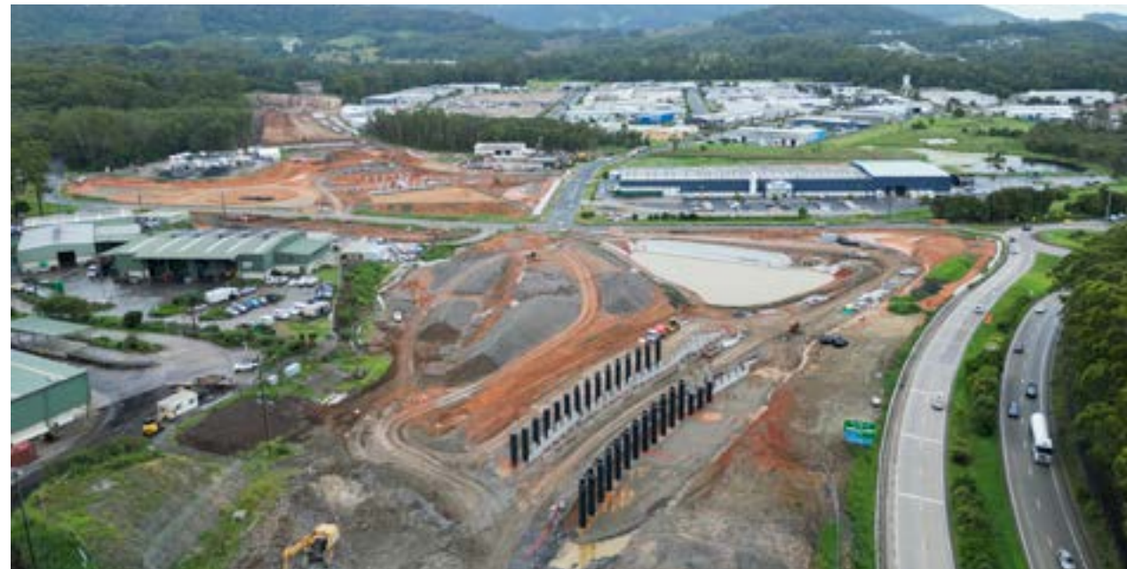
Bridge for off-ramp from the Pacific Highway, south of the Englands Road Interchange, pictured (top) in October 2023 and (bottom) in January 2024.
