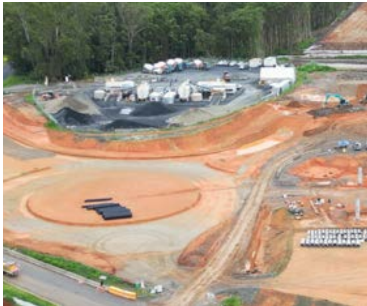
A concrete batch plant pictured (top) in October 2023 and (bottom) in February 2024, has been set up to provide 3.3 million cubic metres of concrete for the project.
