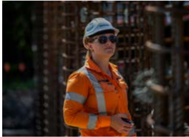
Above: an engineer inspects a bridge column. Right: crane lifting substructure into place for the bridge over North Boambee Road.
