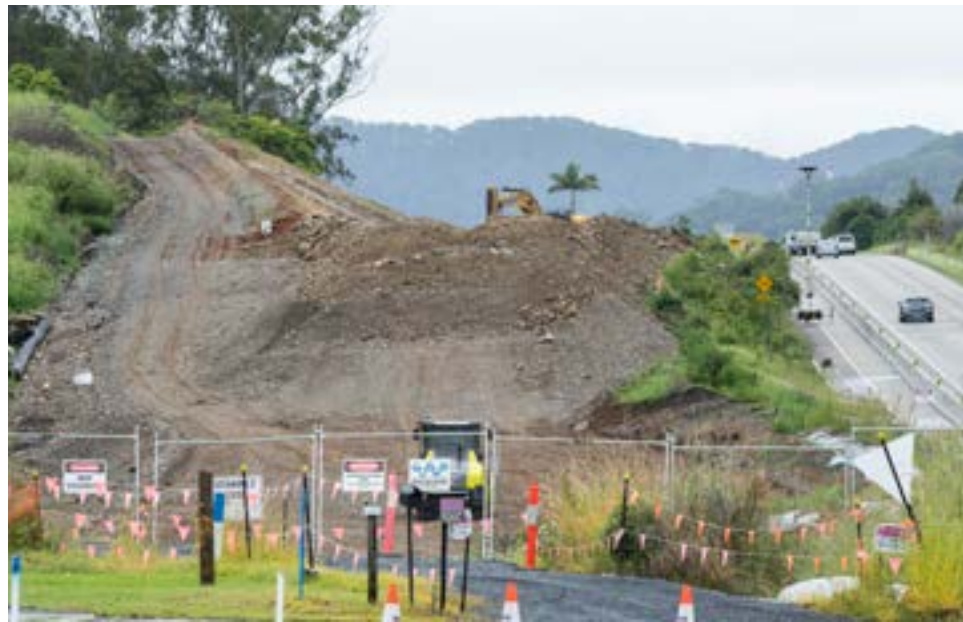
The southern tie-in of the Coffs Harbour bypass with the Pacific Highway near Boambee, pictured (top) in September 2023 and (bottom) in January 2024.
