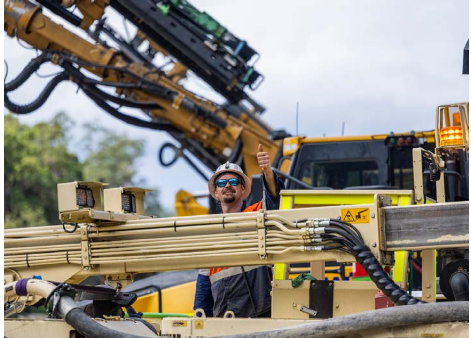
Excitement for the start of tunnelling was felt by the whole team.
