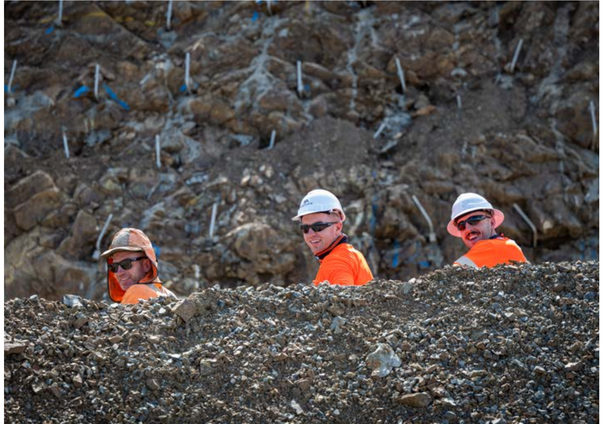
Skilled tradesmen install drainage lines and prepare the steep slope near the deep cut left for shotcreting.
