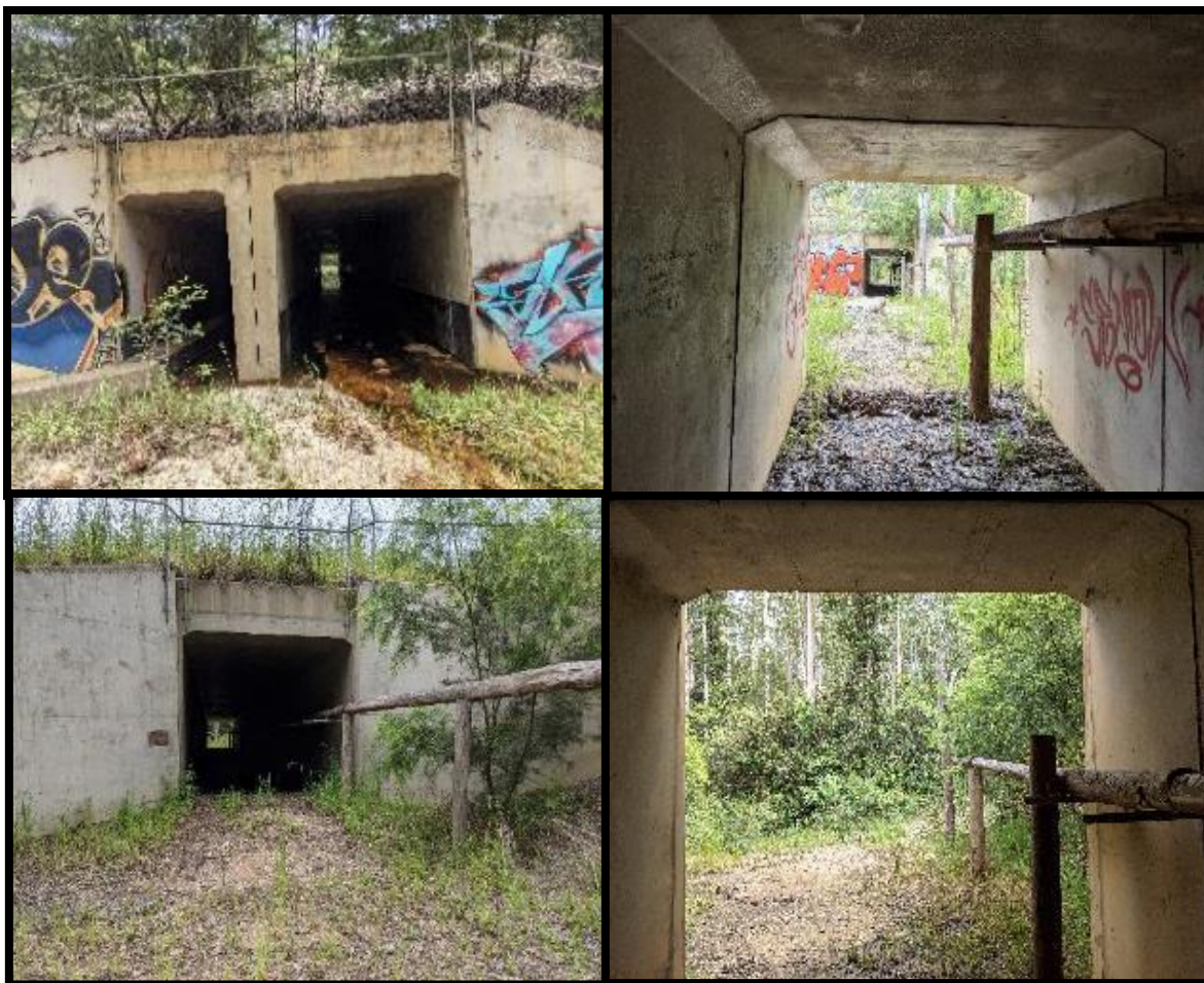
Plate 1. Dual box culverts with designated wet passage at site 5 (top left). Split median box culverts at site 9 and 10 (top right). Fauna furniture entering (bottom left) and exiting site 8 (bottom right).
