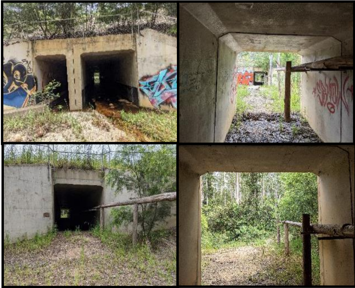
Plate 1. Dual box culverts with designated wet passage at site 5 (top left). Split median box culverts at site 9 and 10 (top right). Fauna furniture entering (bottom left) and exiting site 8 (bottom right).
