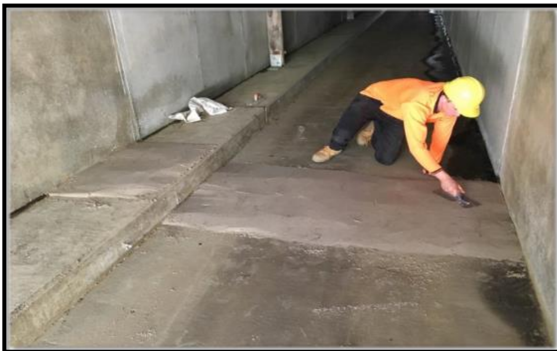
Plate 2. Sand pad being installed in a fauna underpass (Site 3) on the WC2NH upgrade.
