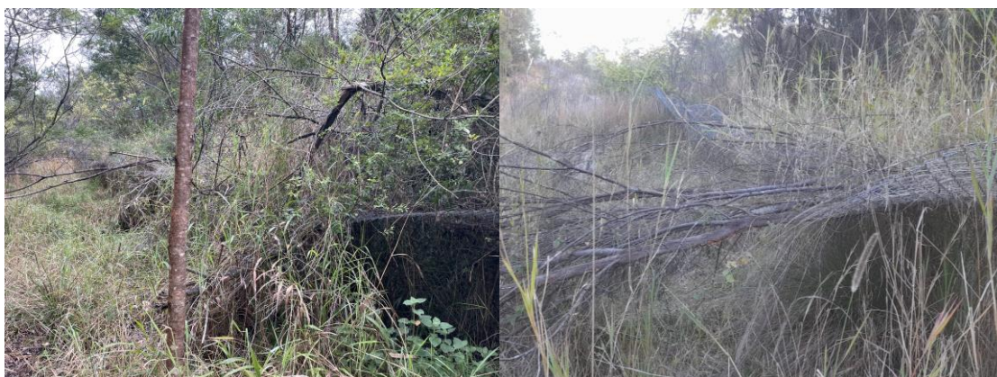
Plate 3: Thick grass protruding through and over the fence (left), and fallen tree/branches onto the fence (right).
