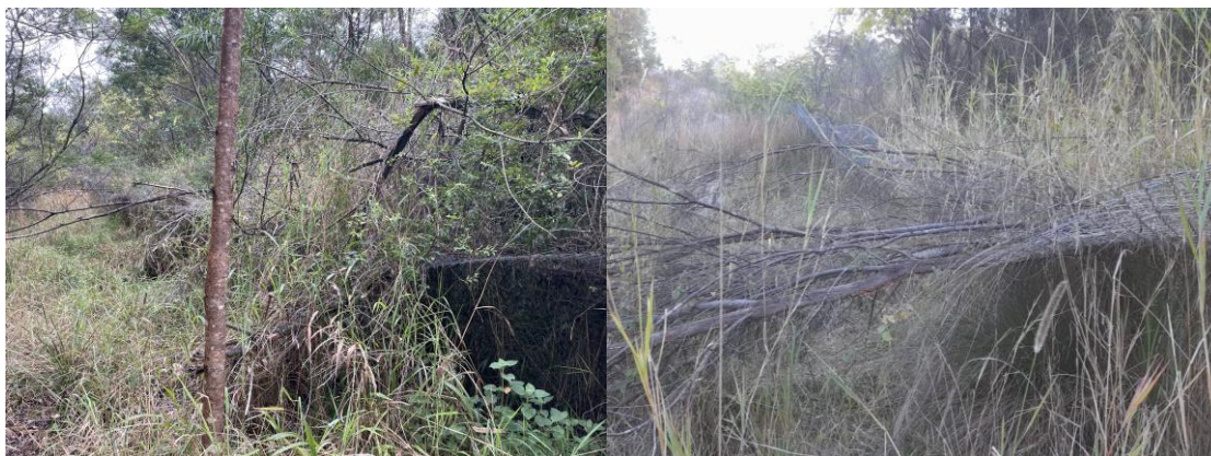
Plate 3: Thick grass protruding through and over the fence (left), and fallen tree/branches onto the fence (right).
